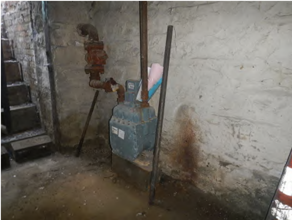
Gas-meter in the basement
