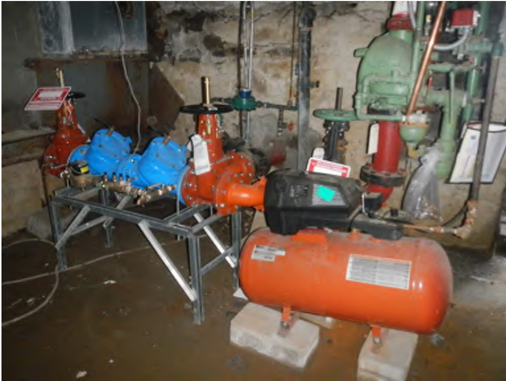
Water meters in the basement
