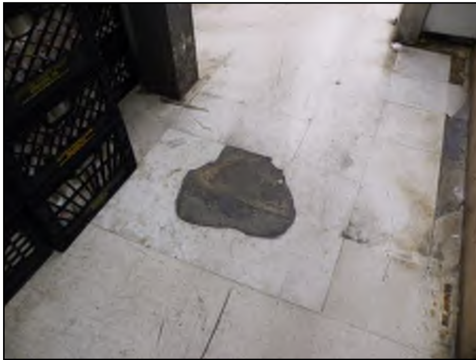
Damaged floor tile
