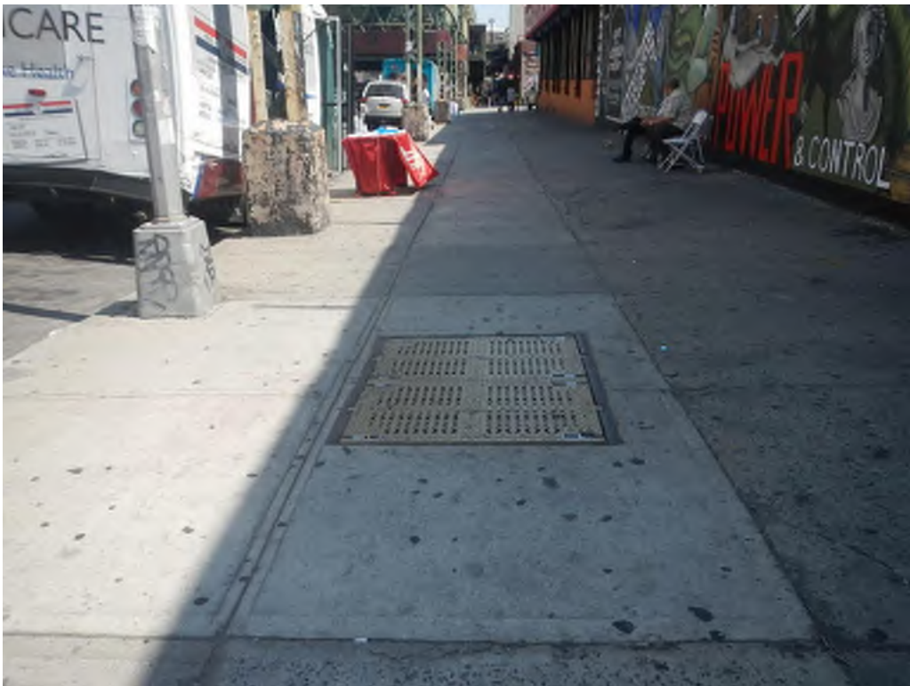
Con Edison vault observed along Myrtle Avenue
