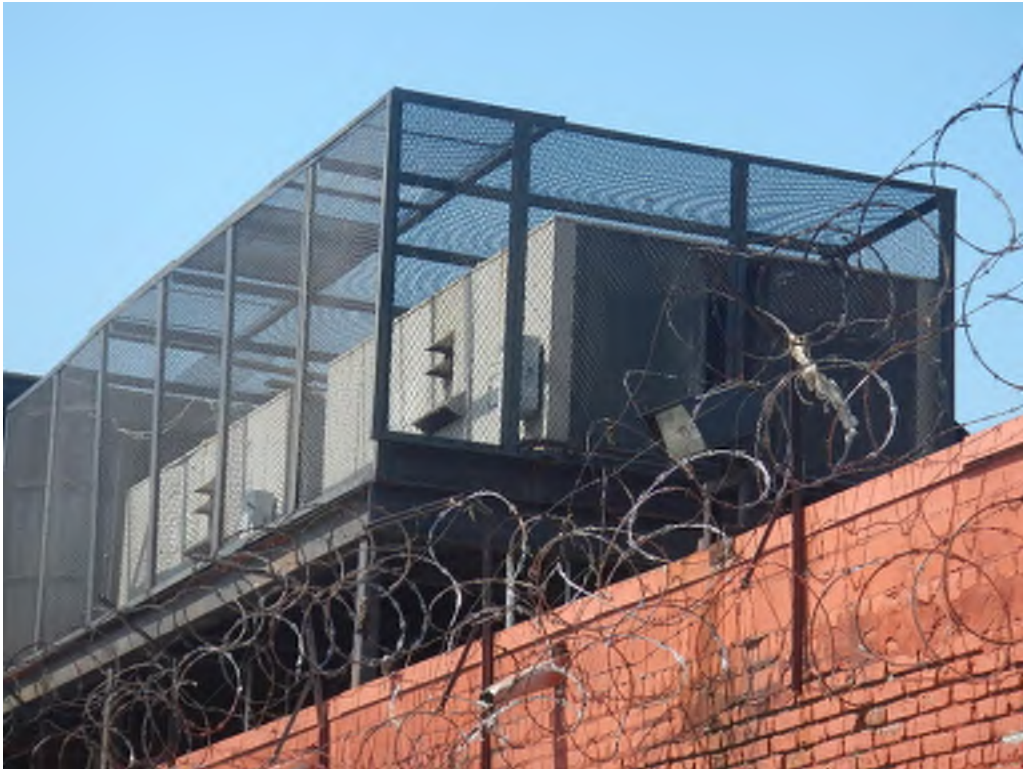
Rooftop mounted HVAC units
