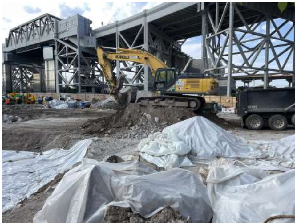
Photo 2: Bauer loading a tri-axle truck with non-hazardous soil for offsite disposal (facing southeast).
