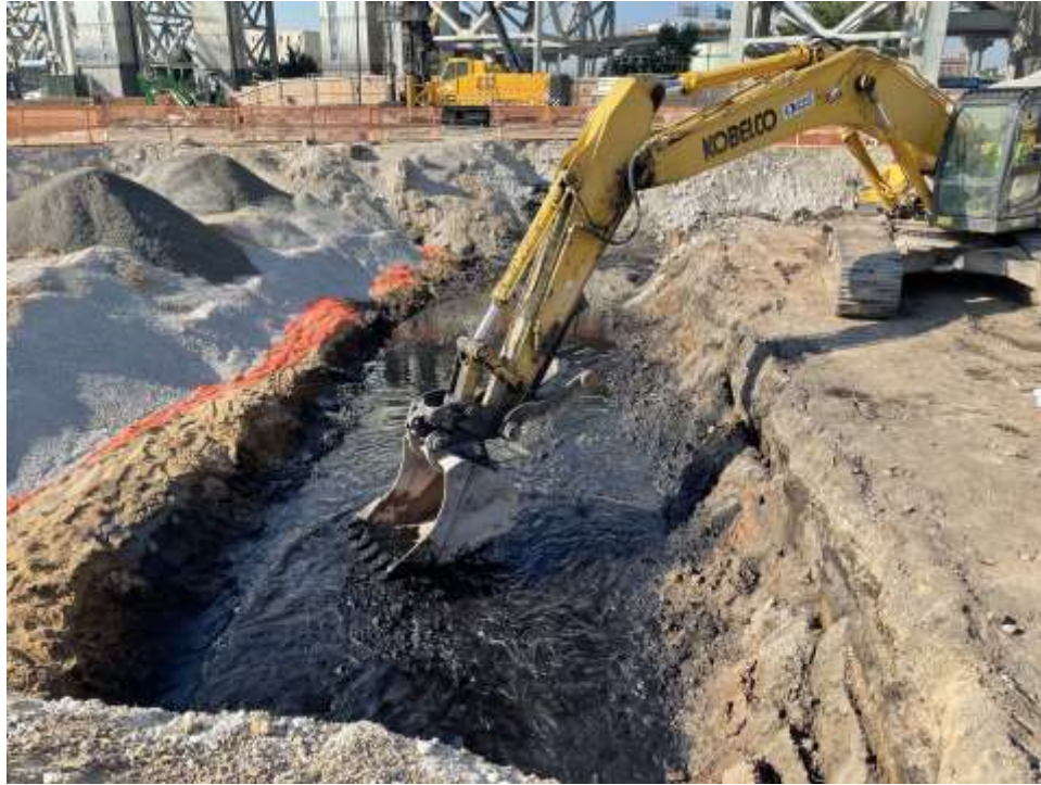
Photo 1: Bauer applying Petro-Fix in the central part of the site (facing east).
