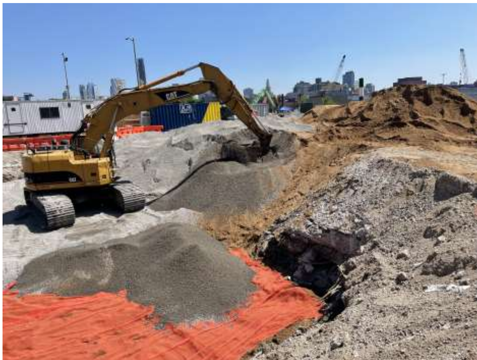
Photo 2: Bauer placing demarcation and backfilling in the central part of the site (facing northeast).
