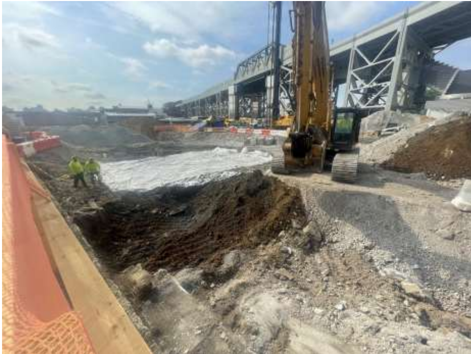
Photo 1: Bauer excavating and stockpiling in the central part of the site (facing southeast).
