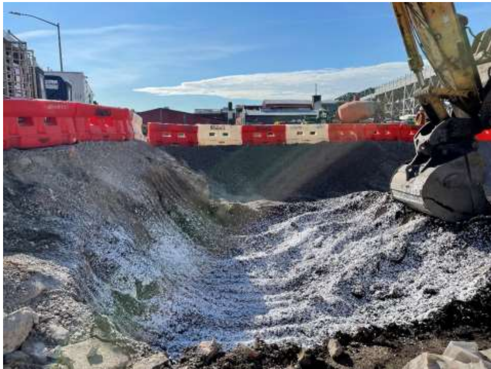
Photo 2: Bauer applying foam in the excavation in the northern area of the site (facing east).
