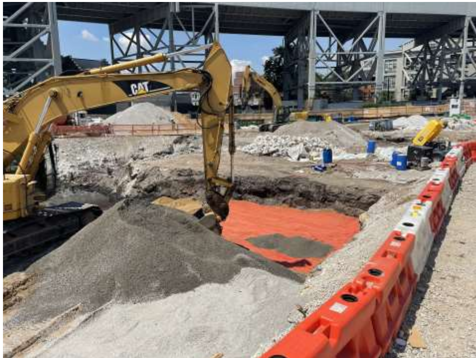
Photo 2: Bauer placing demarcation and backfilling in the central part of the site (facing northeast).
