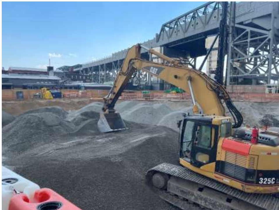
Photo 2: Bauer backfilling with RCA in the eastern part of the site (facing southeast).
