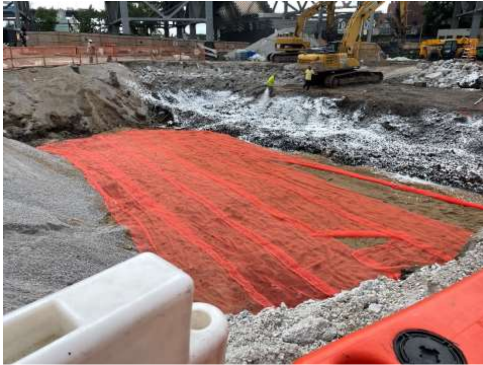
Photo 1: Bauer placing demarcation and applying odor suppressing foam in the northern part of the site (facing southwest).
