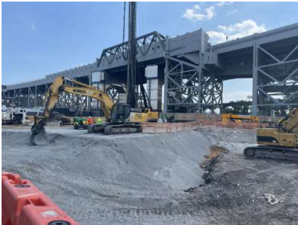
Photo 2: Bauer backfilling with RCA in the eastern part of the site (facing southeast).
