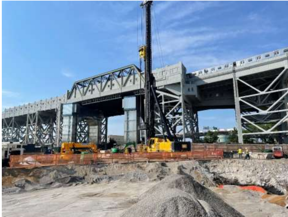
Photo 1: Morris-Shea advancing production piles in the southeastern part of the site (facing south).
