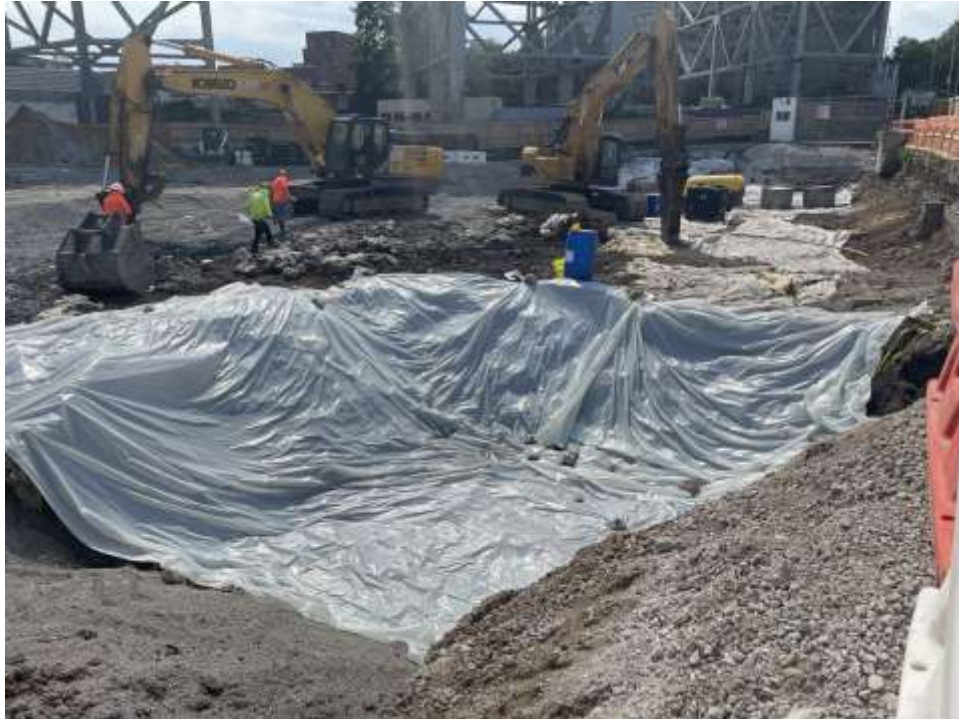
Photo 2: Bauer placing polyethylene sheeting over the excavation in the northern area of the site (facing southwest).
