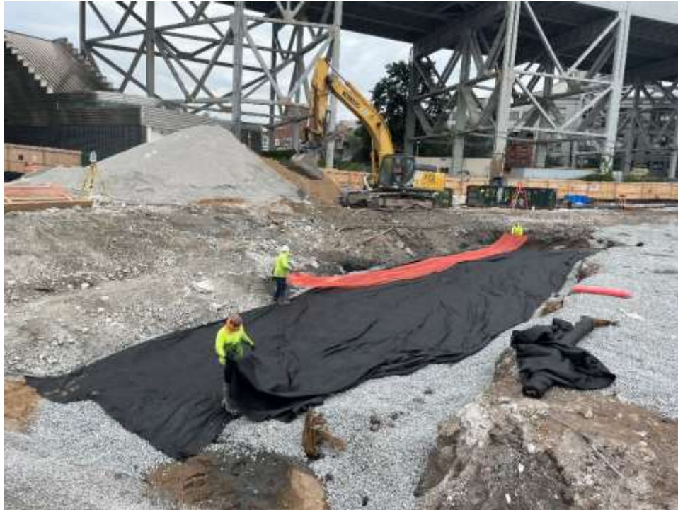
Photo 1: Bauer placing a demarcation layer consisting of Mirafi fabric and orange snow fence within the excavation area (facing southwest).
