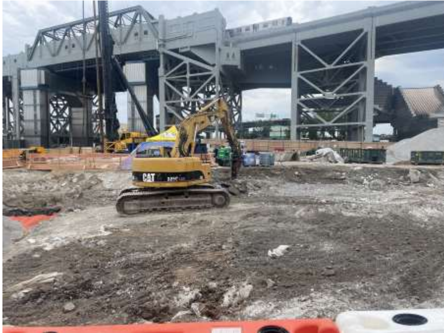
Photo 1: Bauer jackhammering concrete in the southeastern part of the site (facing southeast)
