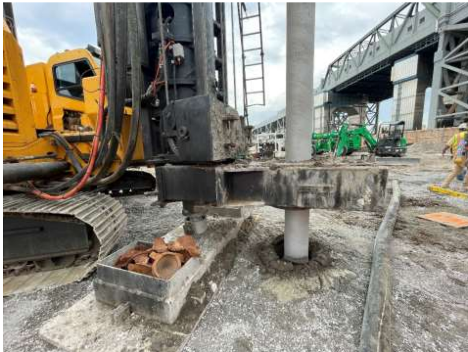
Photo 2: Morris-Shea advancing piles in the eastern part of the site (facing southeast).
