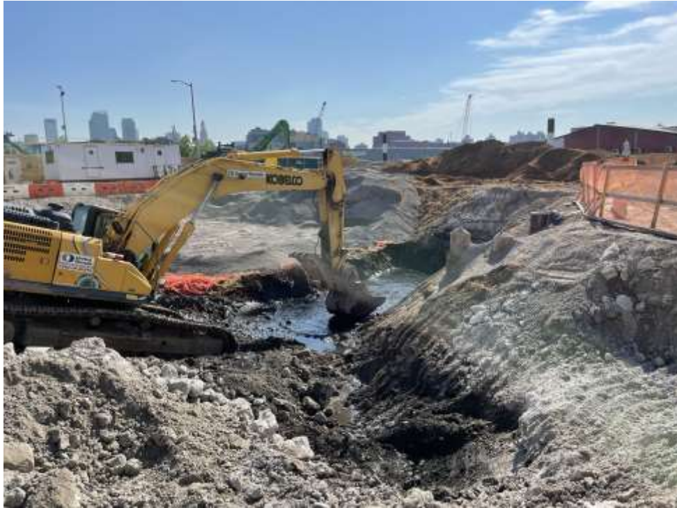
Photo 1: Bauer applying Petro-Fix in the central area of the site (facing east).
