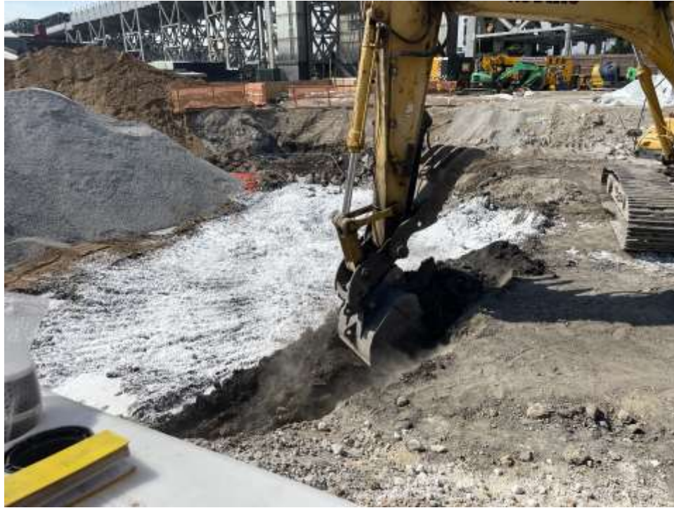
Photo 1: Bauer excavating in the northern part of the site and applying odor suppressing foam to the base of excavation (facing southeast).
