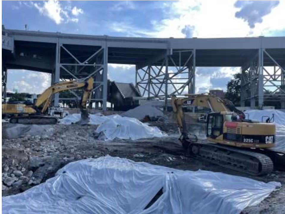
Photo 2: Polyethylene sheeting covering stockpiles and excavation areas across the site (facing southwest).
