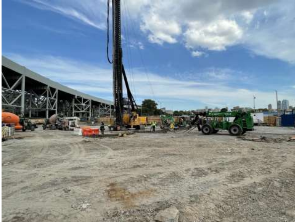
Photo 1: Morris-Shea advancing piles in the central part of the site (facing northwest).
