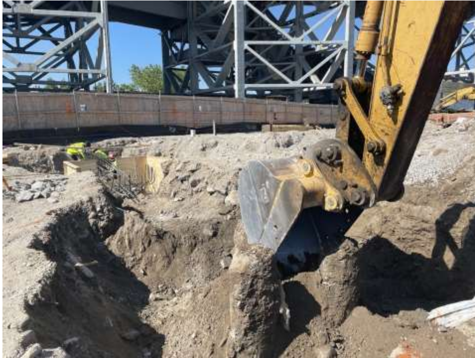
Photo 1: Bauer excavating for pile cap form work installation in the southeastern part of the site (facing southwest).
