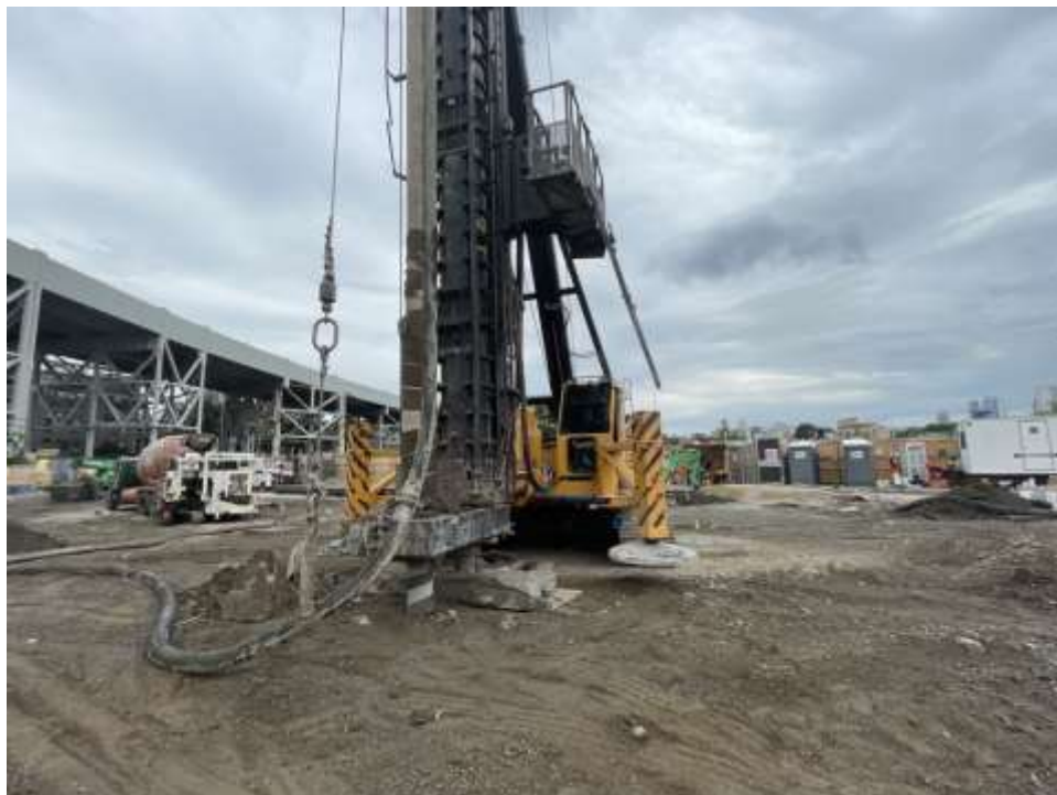
Photo 2: Morris-Shea advancing piles in the central part of the site (facing northwest).
