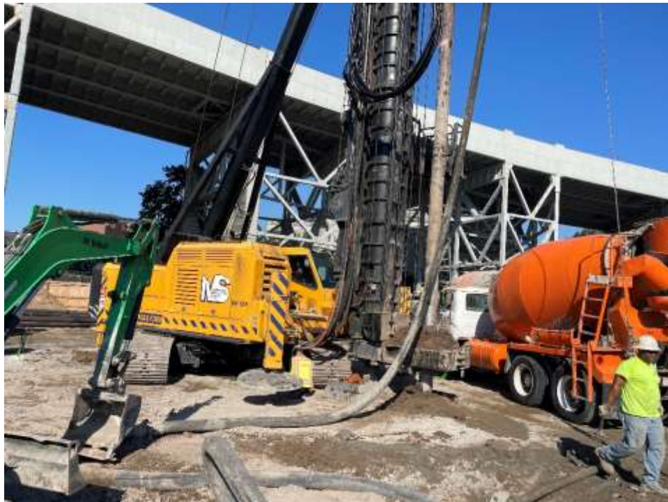
Photo 2: Morris-Shea advancing piles in the central part of the site (facing west).
