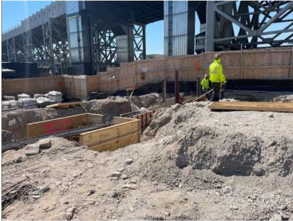
Photo 1: Bauer installing formwork and rebar for pile cap and grade beam installation (facing southeast).
