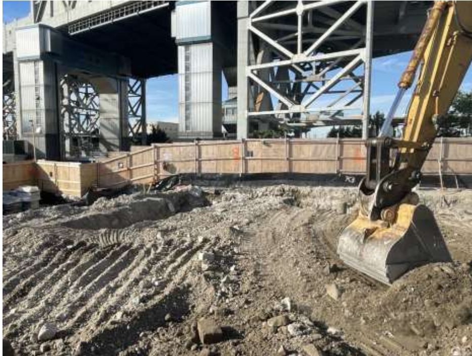
Photo 1: Bauer excavating for pile cap formwork installation in the southeastern area of the site (facing south).
