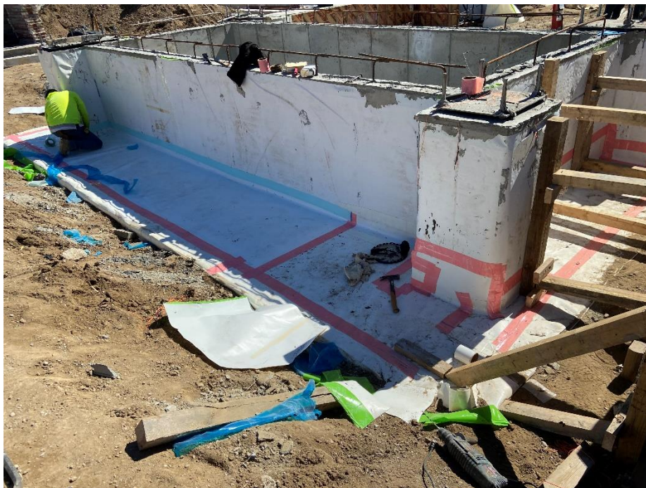
Photo 2: Bauer removing formwork in the central part of the site (facing southeast).
