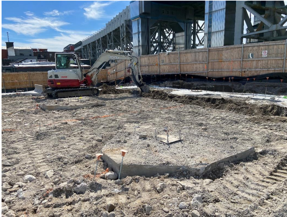
Photo 1: Bauer excavating a shallow trench in the southeastern part of the site in preparation for the installation of the SSDS (facing southeast).
