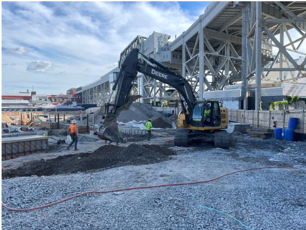
Photo 2: Bauer excavating in the western part of the site in preparation for pile cap formwork installation (facing southeast).
