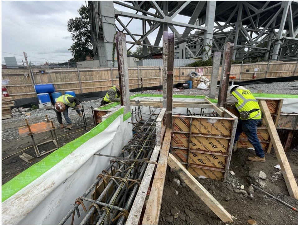
Photo 1: Bauer installing waterproofing/vapor barrier membrane (Preprufe 160R Plus) on the vertical walls within the formwork in the western part of the site (facing west).
