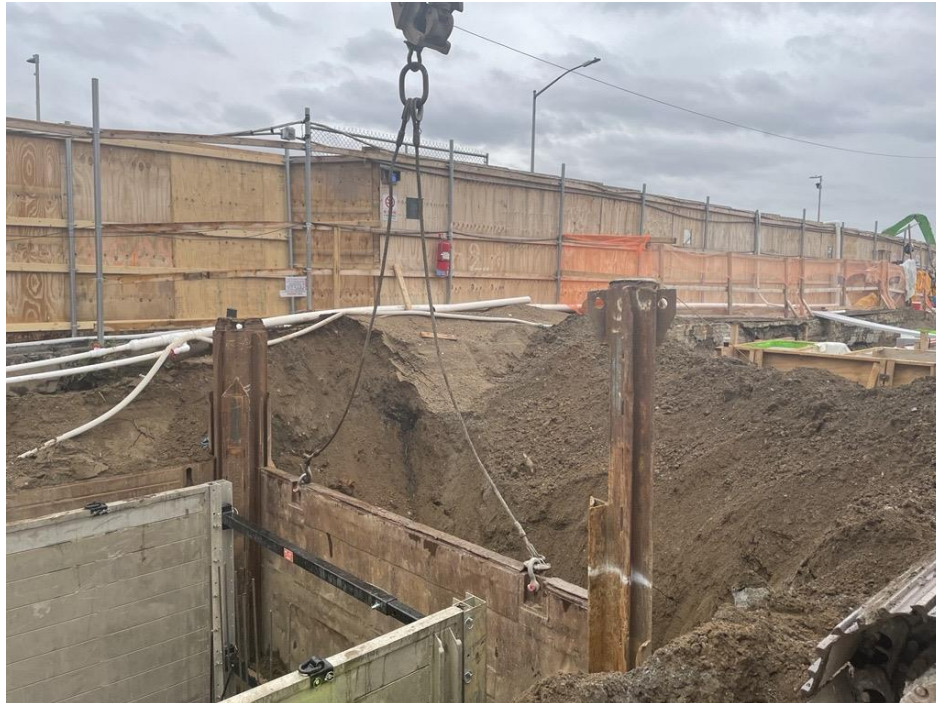
Photo 2: Bauer removing the sides of the shoring box in the northwestern part of the site (facing northeast).
