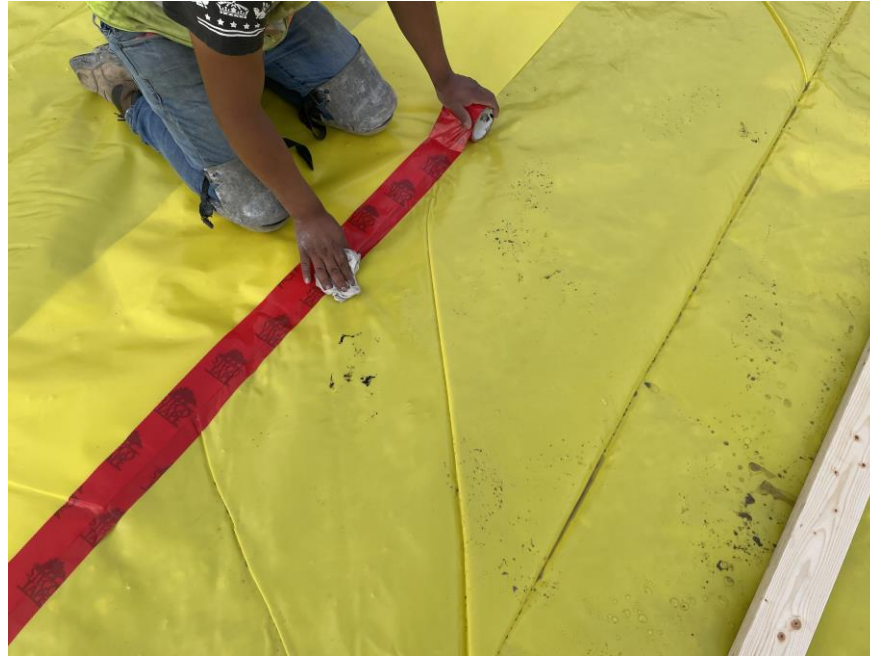
Photo 1: Bauer installing Stego® Wrap 20-mil Vapor Barrier in the northeastern part of the site (facing down).
