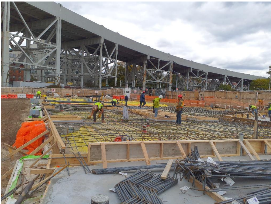
Photo 2: Bauer installing rebar reinforcement for the SMD system in the western part of the site (facing west).
