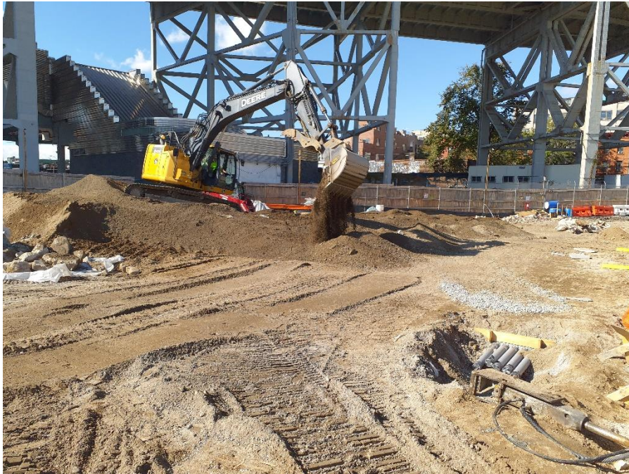
Photo 1: Bauer backfilling the southern part of the site with RCA/clean fill (facing southwest).
