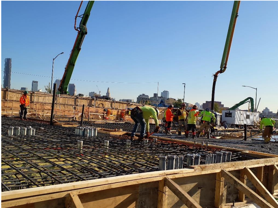
Photo 1: Bauer pouring concrete for the foundation slab in the western part of the site (facing northeast).
