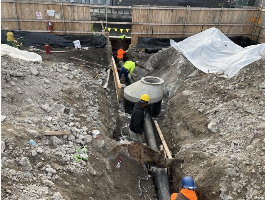
Photo 1: American Standard installing the stormwater sewer in the southeastern part of the site (facing east)
