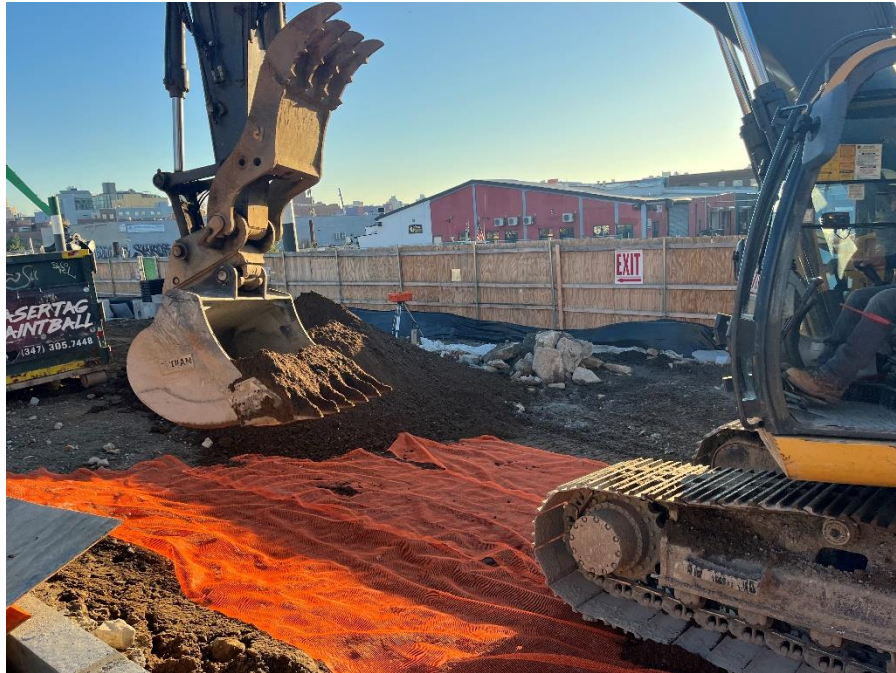
Photo 1: Bauer placing imported fill on top of the demarcation layer in the southeastern part of the site (facing northeast)
