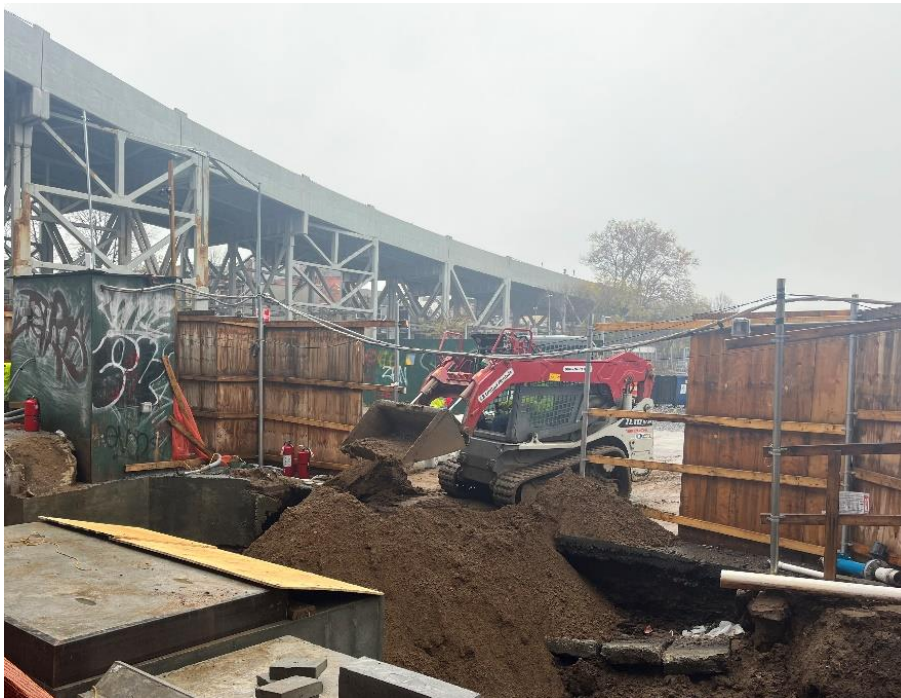
Photo 2: Bauer stockpiling imported clean fill from EROC in the northwestern part of the site (facing northwest)
