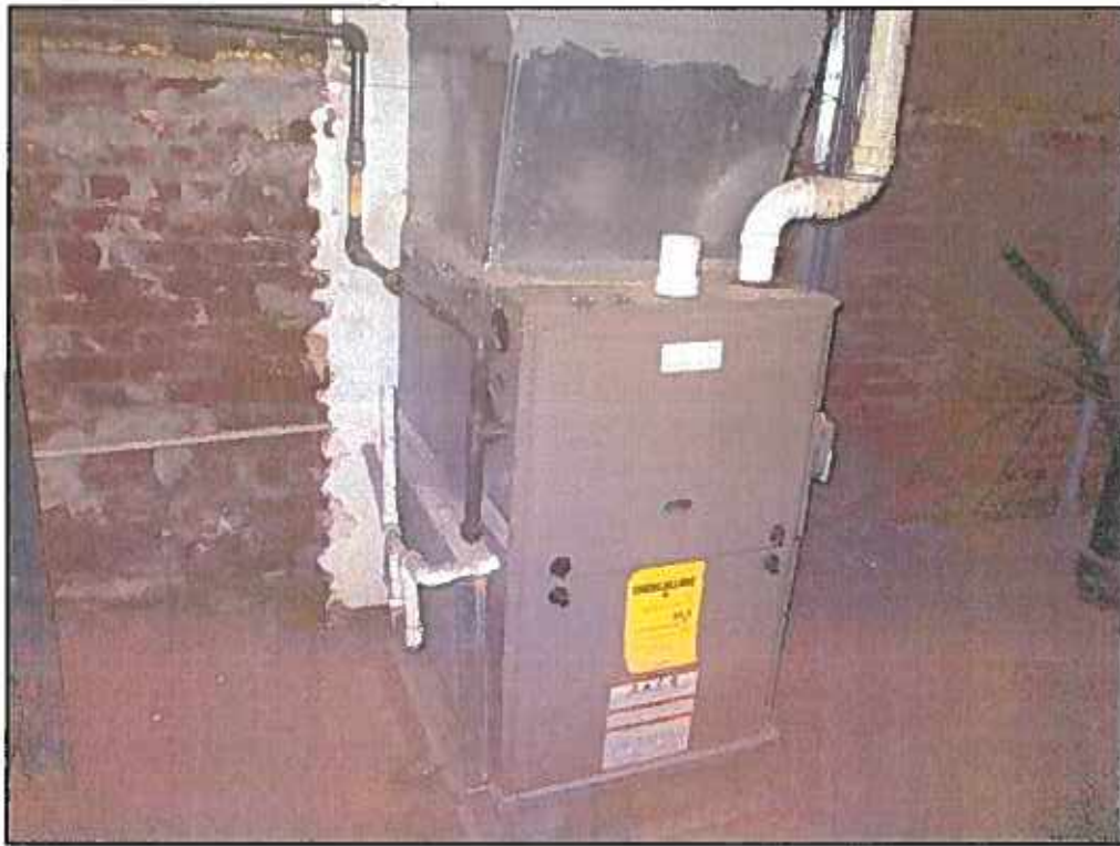
35 : View of the natural gas fired boiler in the basement of 253 Bond Street.
