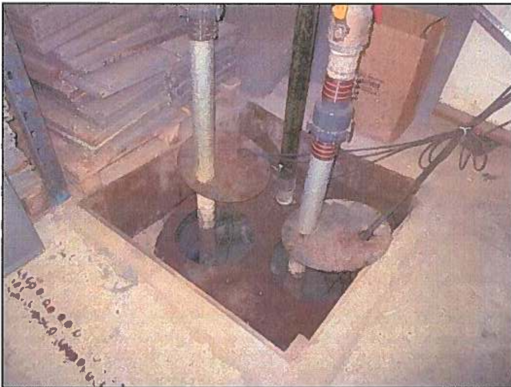
34 : View of a sump pump within the basement at 253 Bond Street.
