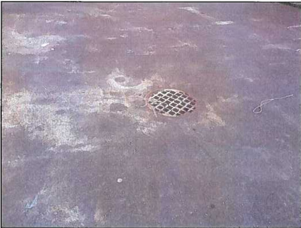
30 : View of a stormwater inlet within the loading area at 253 Bond Street.
