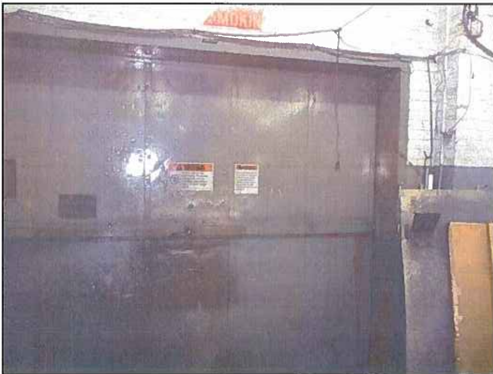
38 : View of the cable pulley freight elevator at 253 Bond Street.
