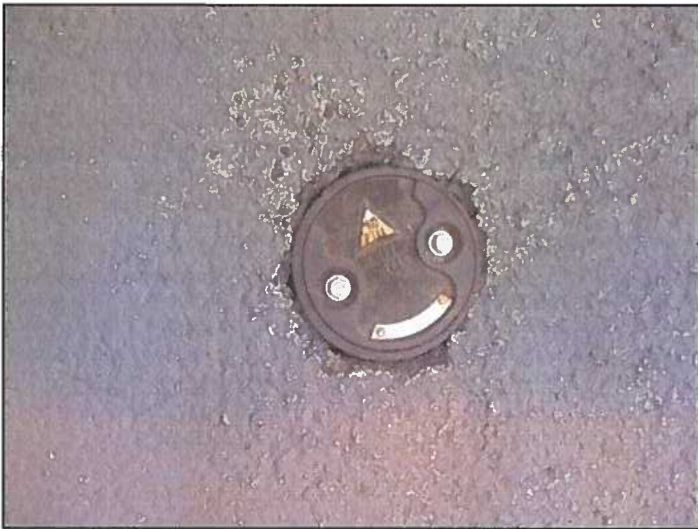
29 : View of a monitoring well within the loading area at 253 Bond Street.
