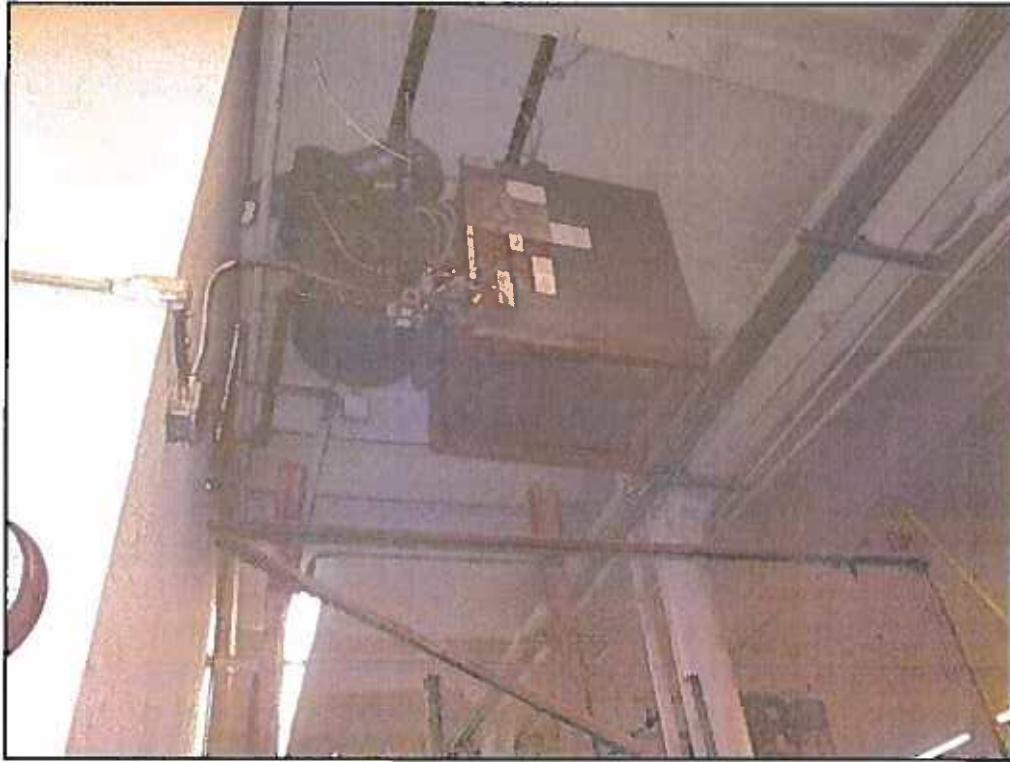
43 : View of the heating unit mounted to the ceiling on the first floor of the warehouse at 253 Bond Street.
