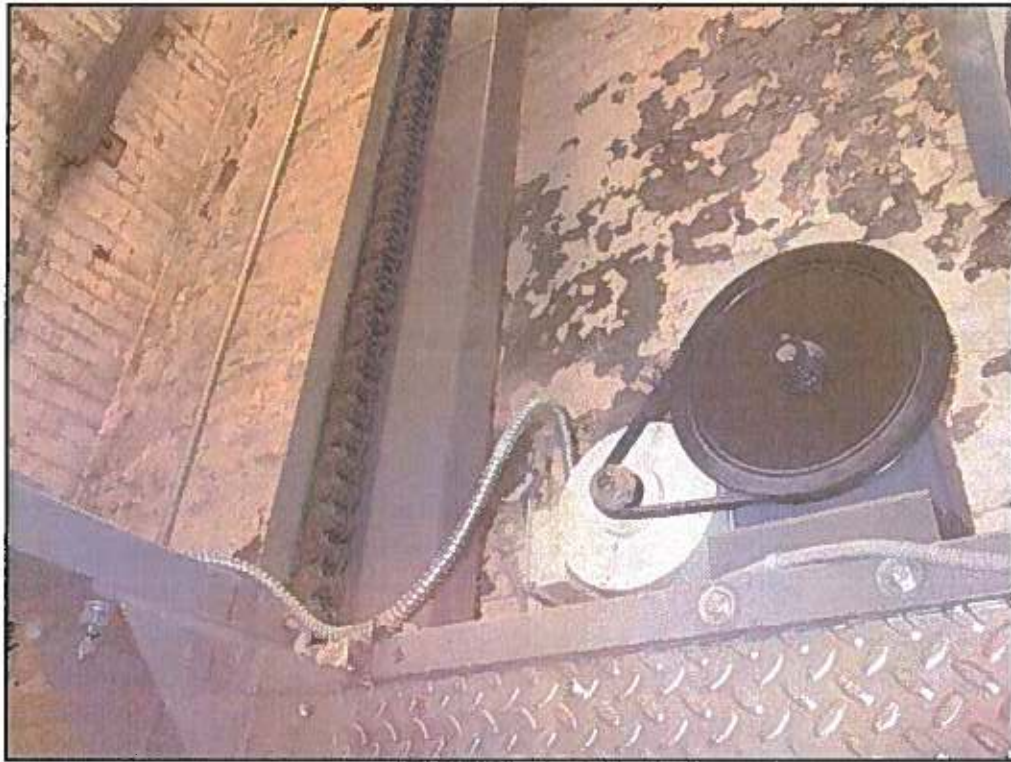
39 : View of the elevator pulley system within the elevator shaft (note peeling paint).
