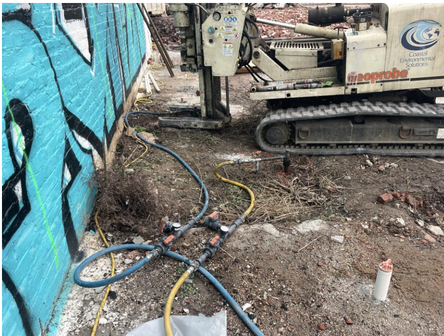
Photo 2: Regensis applying remedial products at injection points IP39A and IP40 (facing east).
