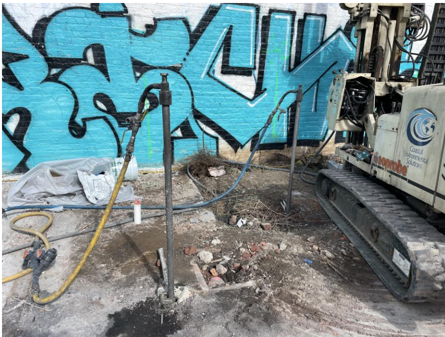
Photo 2: Regensis applying remedial products at injection points IP39B and IP39A (facing north).
