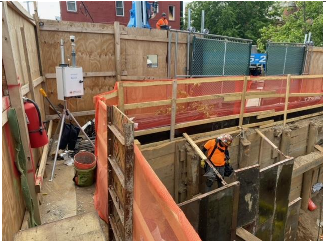
Photo 2 – Facing West Installing forms for western wall. CAMP Station 1 located on SW corner
