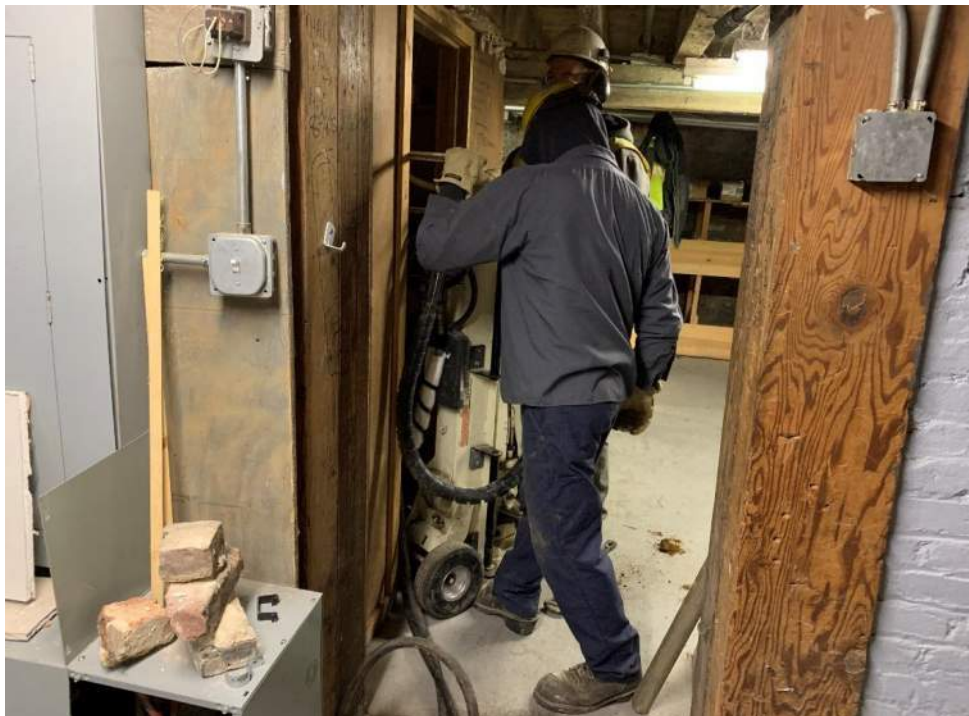
Photograph 9: View of Eastern drilling a soil boring with the Geoprobe® 420M in the cellar portion of the site. Photo taken on January 29, 2020.
