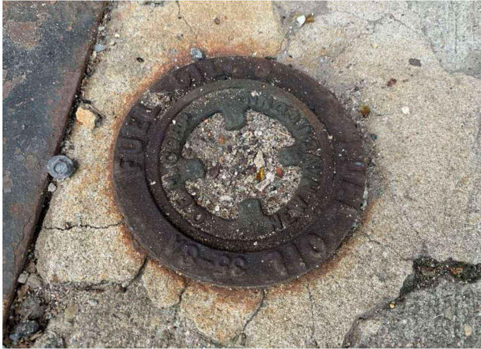
Photograph 7: View of fuel oil fill port located on Rockaway Avenue sidewalk. Photo taken on January 28, 2020.
