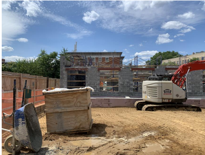
Photo 1: View of backfilled and compacted clean sand in the south-central part of the site (facing west).
