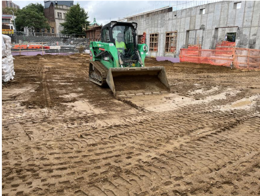
Photo 1: View of Legacy grading clean sand in the central part of the site (facing northeast) .
