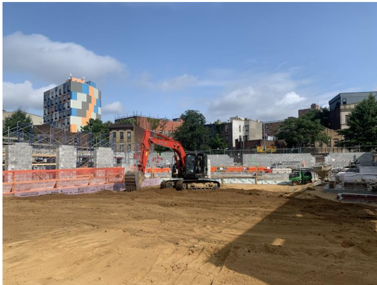
Photo 1: View of Legacy backfilling clean sand in the central part of the site (facing northwest) .
