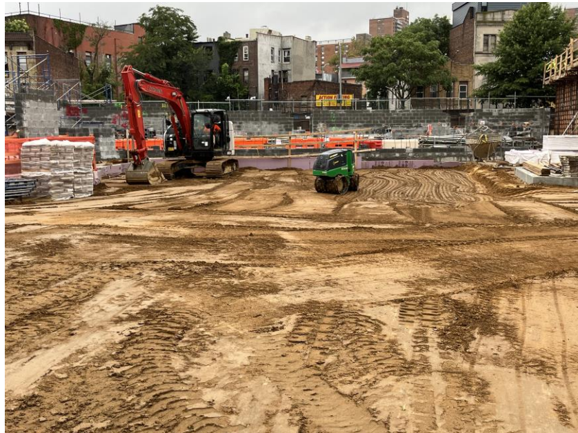
Photo 2: View of Legacy compacting clean sand in the central part of the site (facing north).
