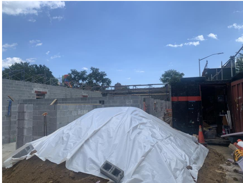
Photo 2: View of clean sand stockpile covered with polyethylene sheeting in the northwestern part of the site (facing south).
