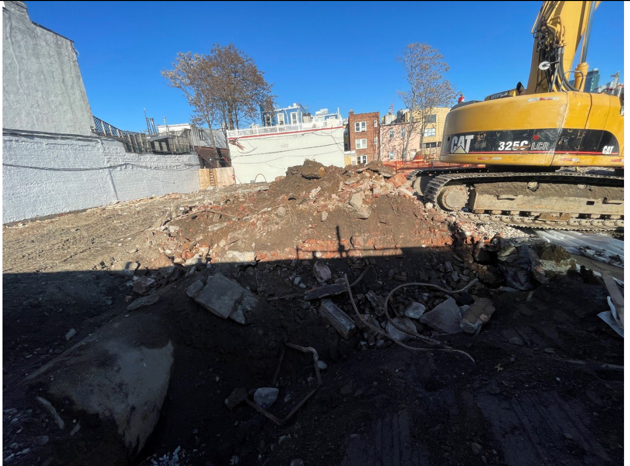
Photo 4 – Representative view of mixed masonry material from WC-6 being loaded out for off-Site disposal at Bayshore.
