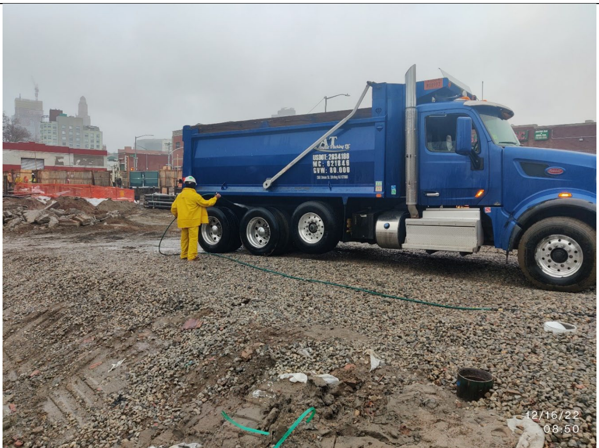
Photo 4 – Representative view of Raptor flagger tire washing, prior to the truck exiting the Site.
