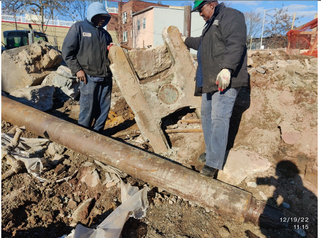
Photo 12- Represneave view of one (1) of the two (2) hydraulic lifts, this lift could not be opened, ABC presumed it empty.
