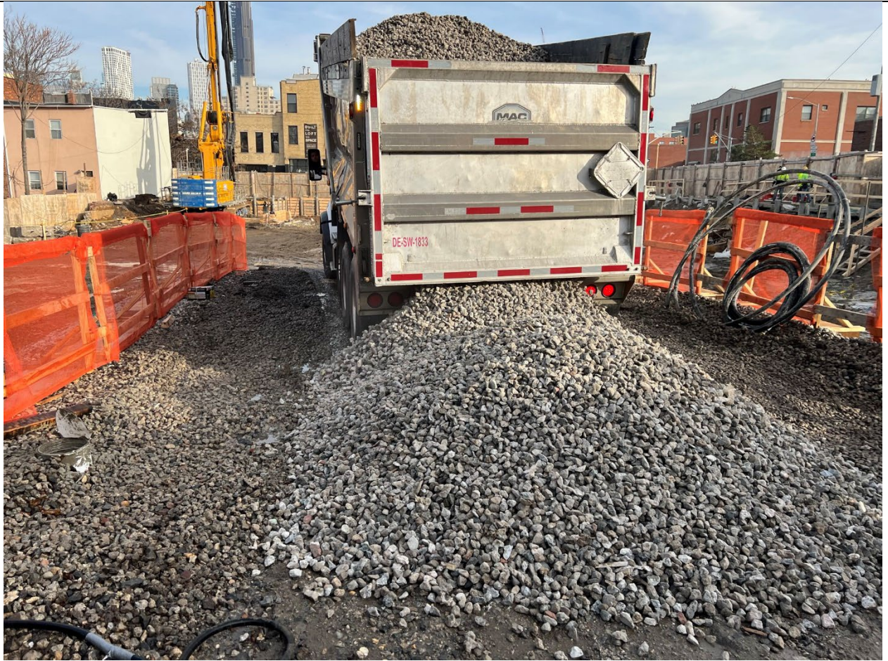
Photo 1 – Representative photo of stone being delivered for the trucking pad at Site truck entrance/exit.
