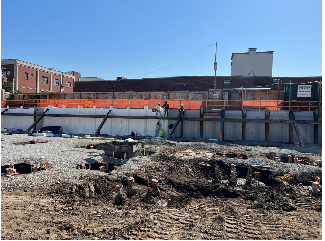
Photo 3 – Representative photo of foam boards and poly being placed against the lagging along 3 rd Avenue.
