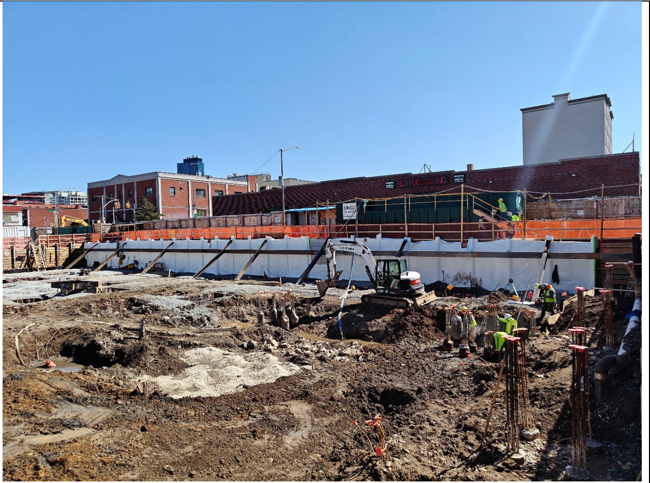
Photo 2 – Attempted excavation work proximal to EP-20, excavation ceased due to issues with dewatering.
