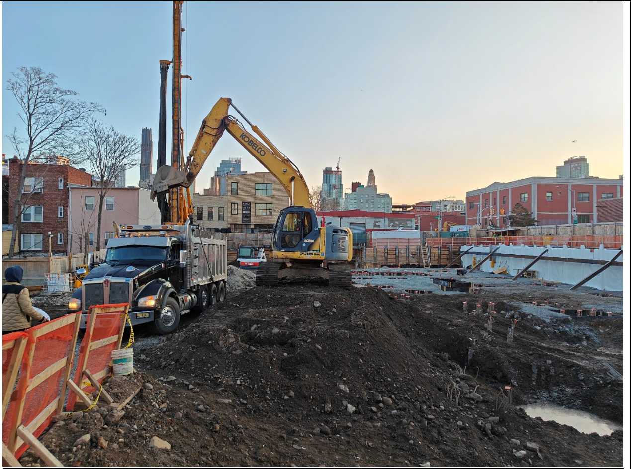
Photo 1 – Representative view of the site at the start of the days activities with soil loading for off- site disposal.
