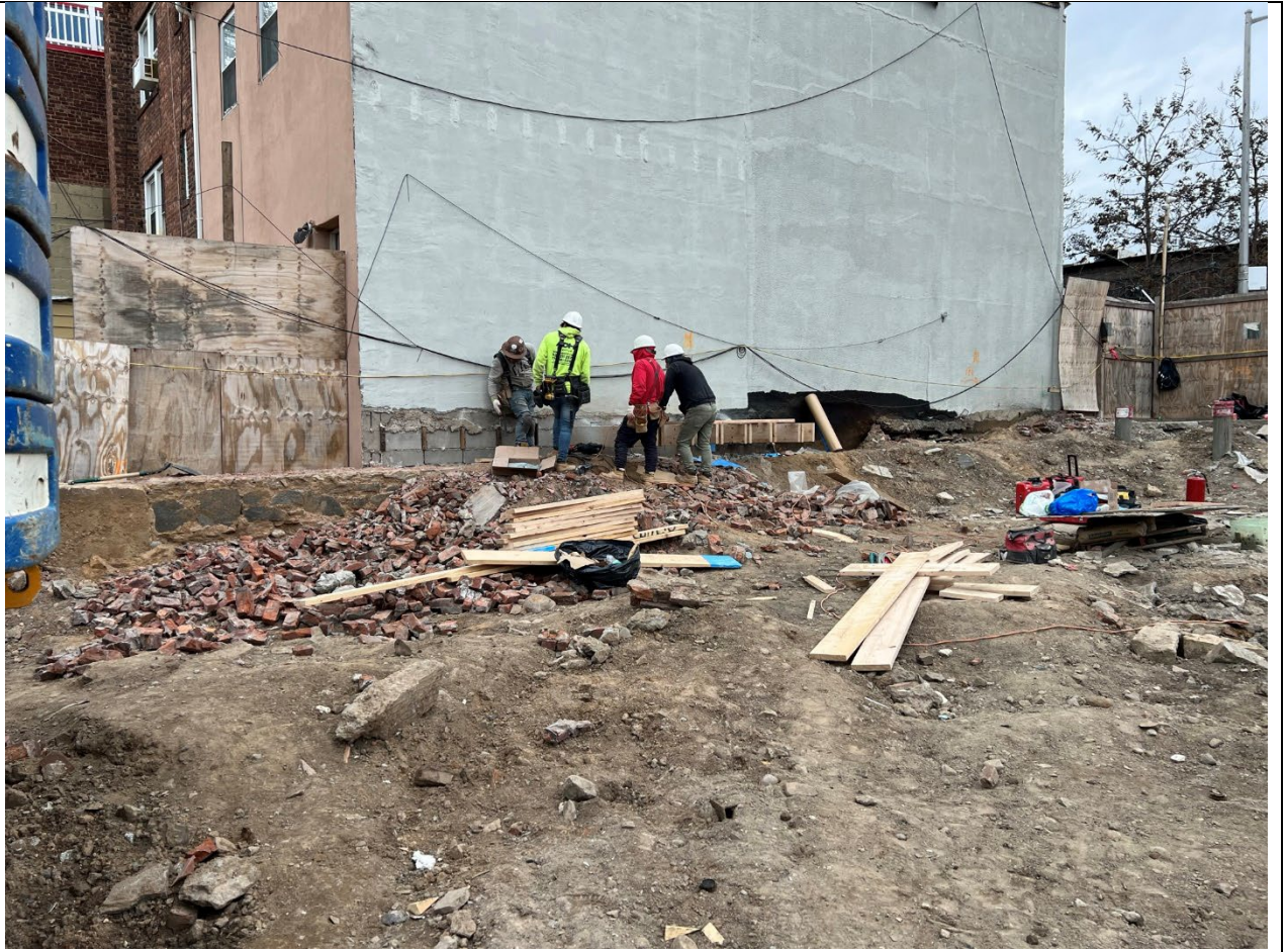
Photo 3 – Representative view of workers fixing the adjacent building located along Sackett Street.
