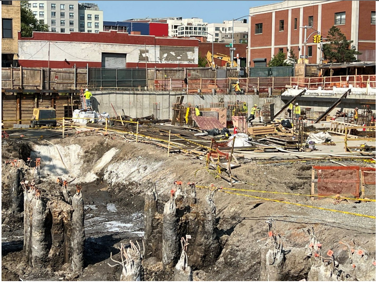
Photo 3 – Representative view of forms being removed from walls on Sackett and 3 rd Avenue.
