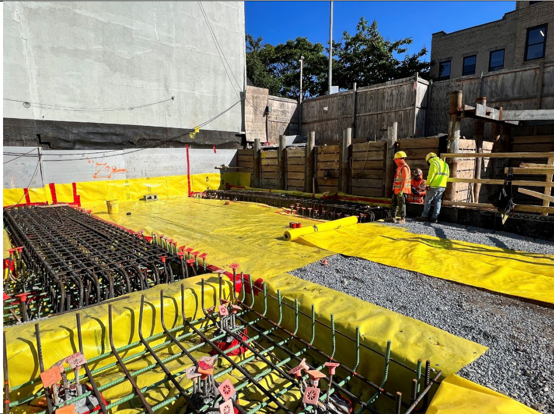
Photo 3 - Representative photo of rebar and vapor barrier work in WC-6 and WC- 7.
