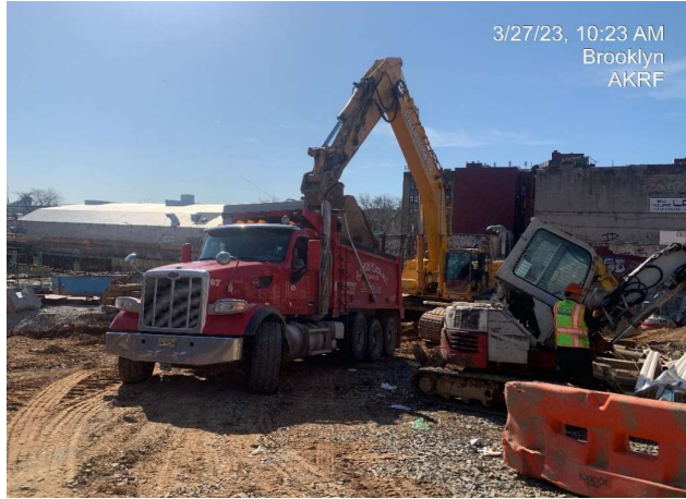
Photograph 1 - Loading soil/fill on to trucks for off-site disposal at the Bayshore Soil Management facility, view facing southwest.
