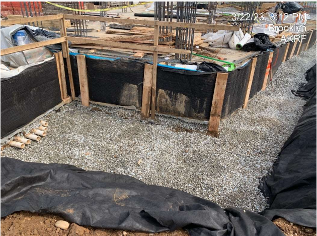
Photograph 3 - Installed GPA as part of the SSDS installation, view facing south.
