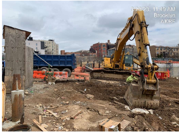
Photograph 1 - Loading soil/fill on to trucks for off-site disposal at the Bayshore Soil Management facility, view facing north.
