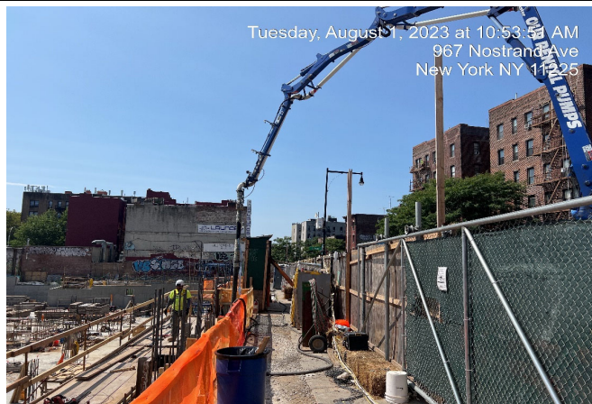
Photograph 3 - Pouring concrete for the western foundation wall in Grids 3 and 7, view facing south.
