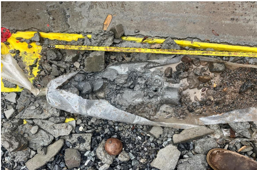
Photo 2: View of soil boring material from the installation of IW-4, facing north.
