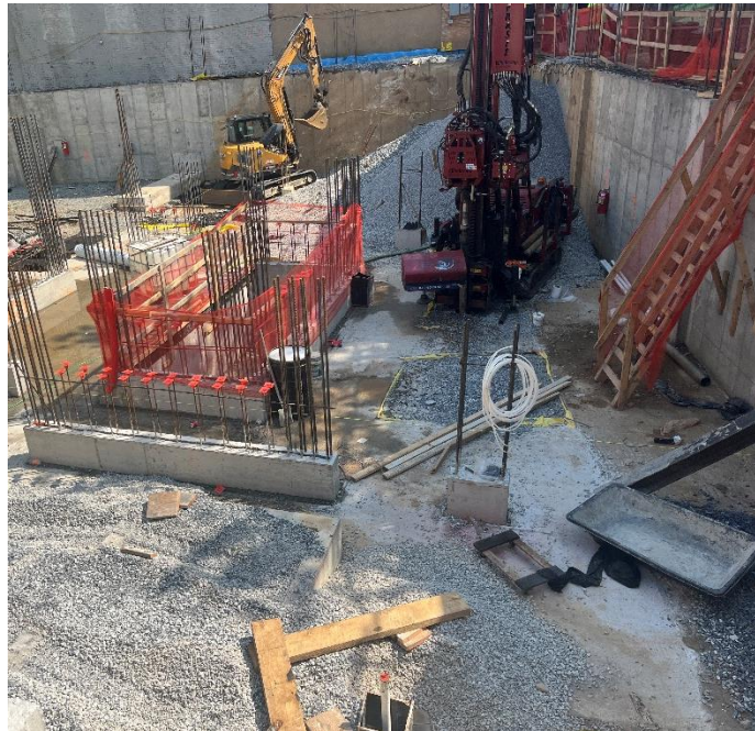
Photo 4: View of Site conditions and installation of injection well IW-04, facing south.
