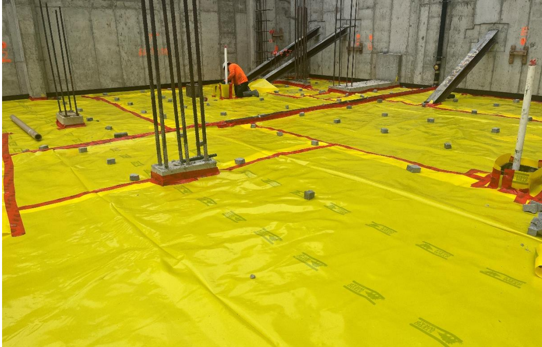
Photo 3: View of the contractor installing the vapor barrier for the SSDS, facing northeast.
