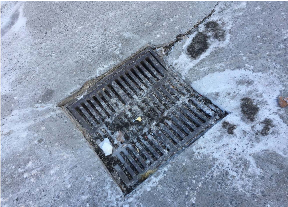
Photograph 6: View of a storm drain located on the subject property, adjacent south of Tillary Street.
