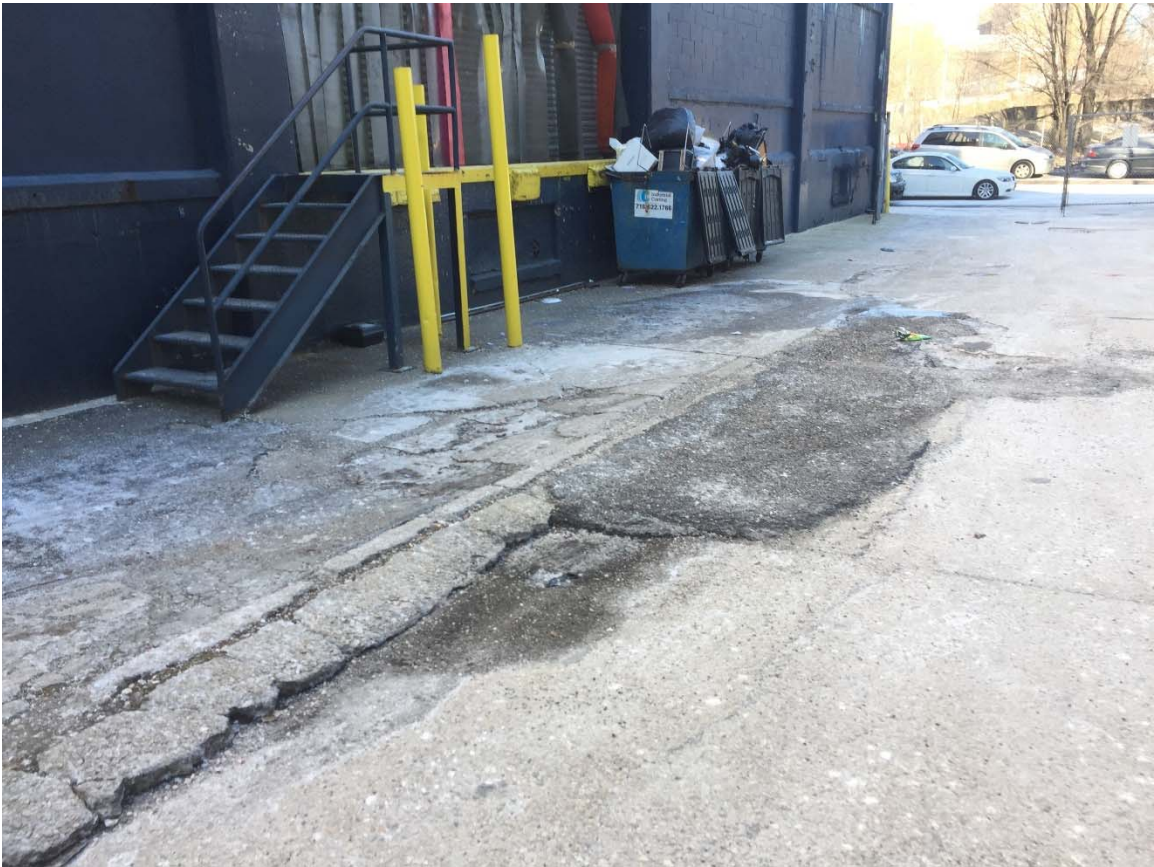
Photograph 7: View of the dumpster area and uneven pavement, facing northwest.
