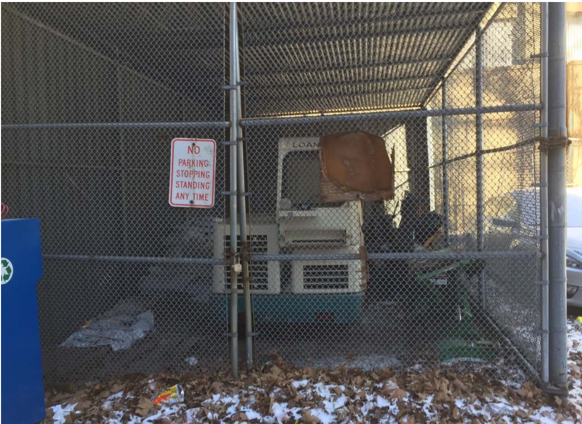
Photograph 10: View of the locked chain-link fence storage enclosure located along the southern boundary of the site, facing north.
