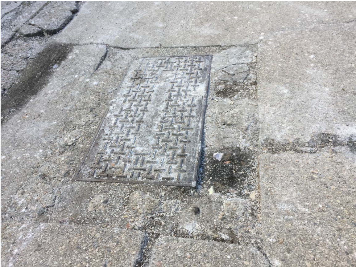
Photograph 8: View of a access plate in the concrete pavement with an unknown origin and use.
