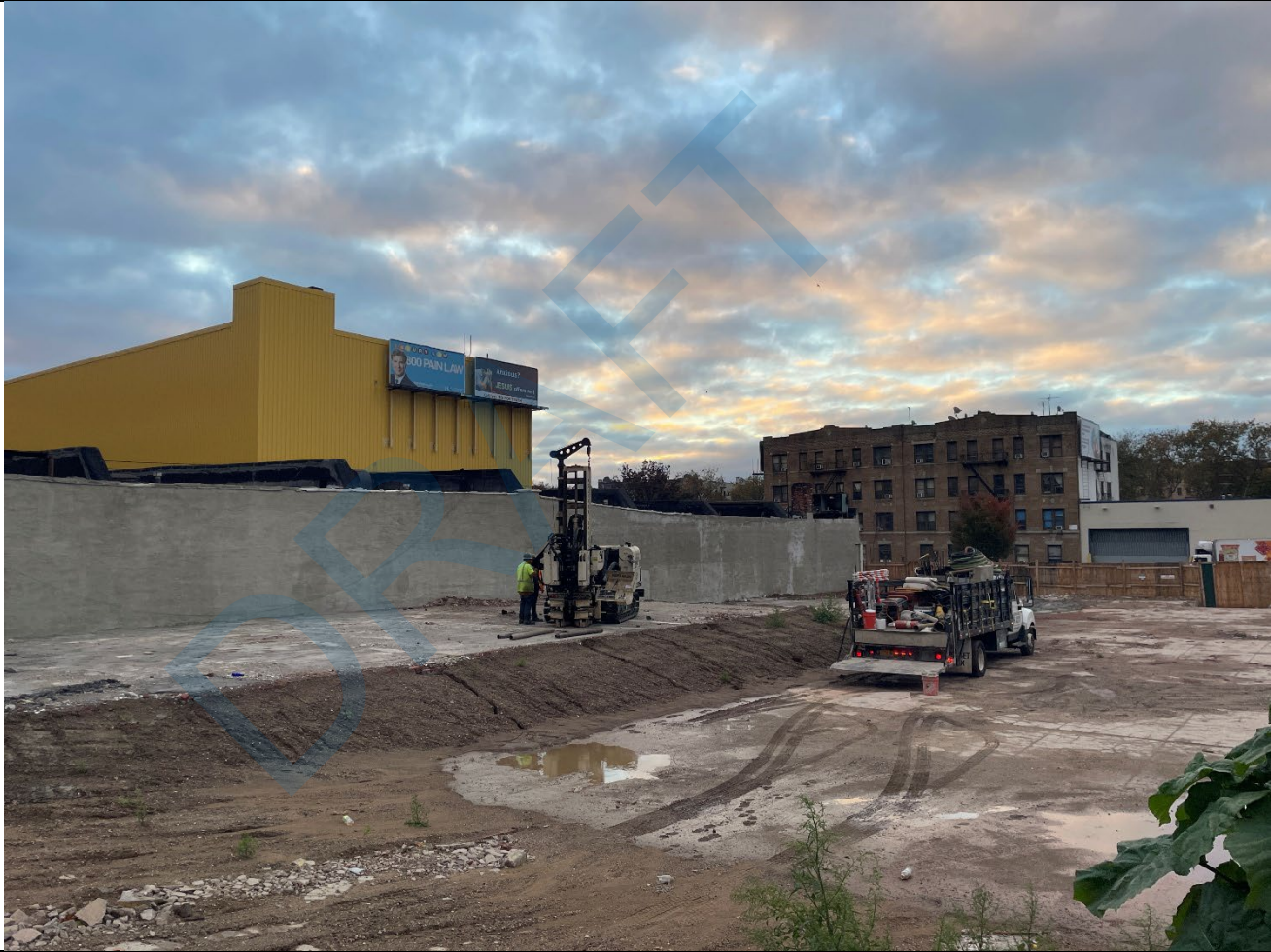
Photo 1: Looking southeast; view of ADT staged at SRI-4.
