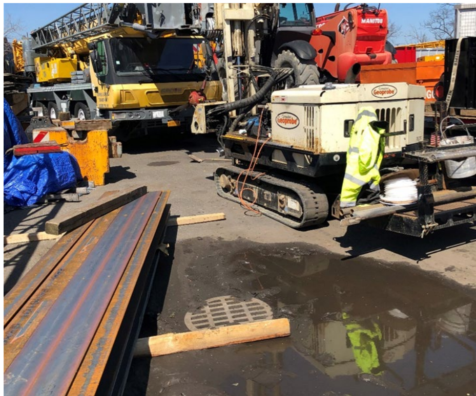
Photograph 7: Impacted storm drain.
