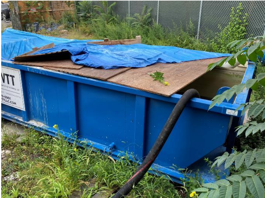
Photo 1: Liquid being pumped from a settling tank into a vacuum truck for off-site disposal (facing southwest)
