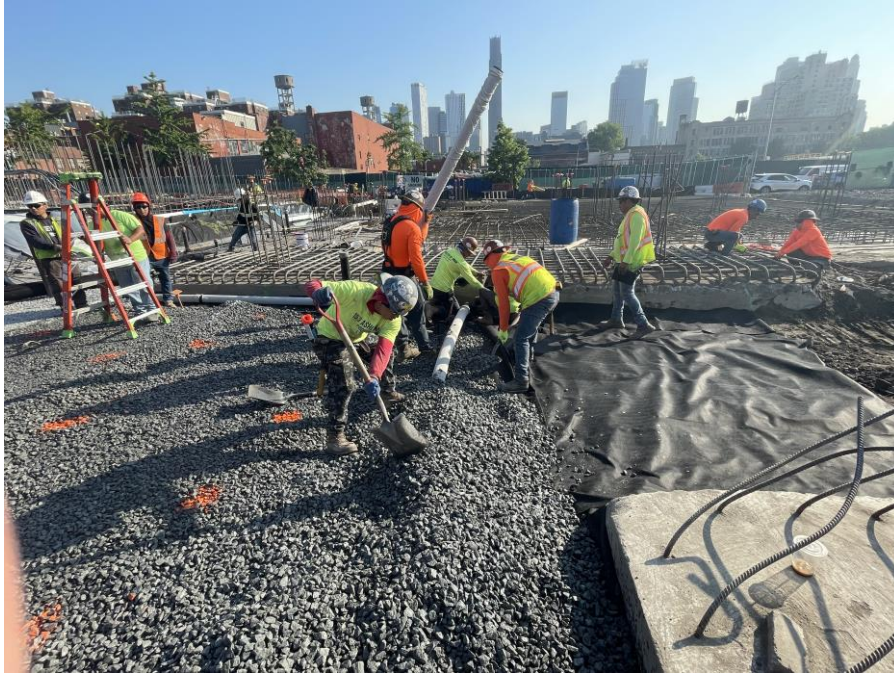
Photo 1: Kingdom installing SMD system components in the northeastern part of Society Brooklyn (facing west)
