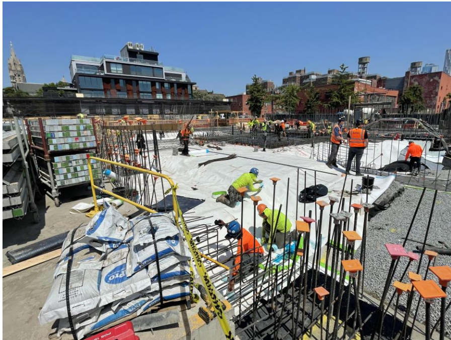
Photo 2: Kingdom installing a waterproofing/vapor barrier membrane in the central part of Society Brooklyn (facing northeast)
