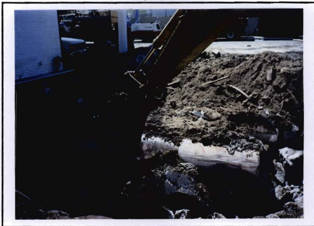
Two 4,000-gallon gasoline underground storage tanks
