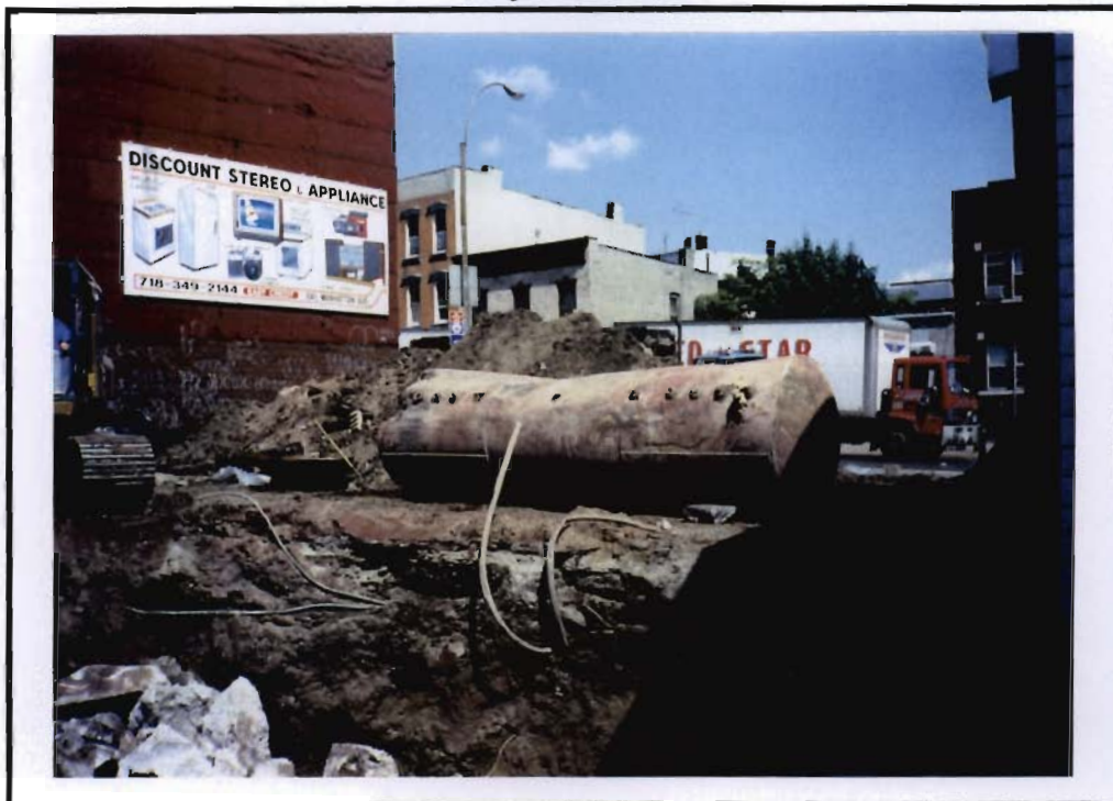
One 4,000-gallon gasoline underground storage tank
