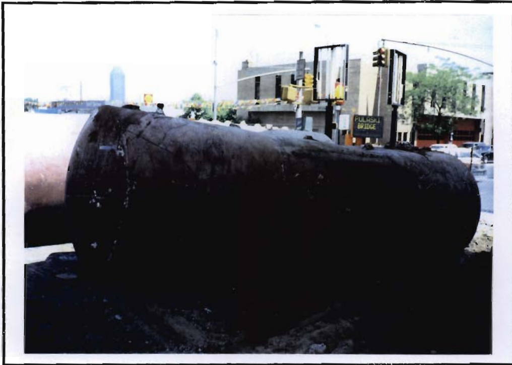
One 4,000-gallon and two 2,000-gallon, gasoline underground storage tanks
