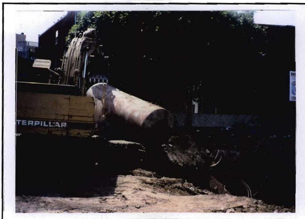
One 4,000-gallon gasoline underground storage tank
