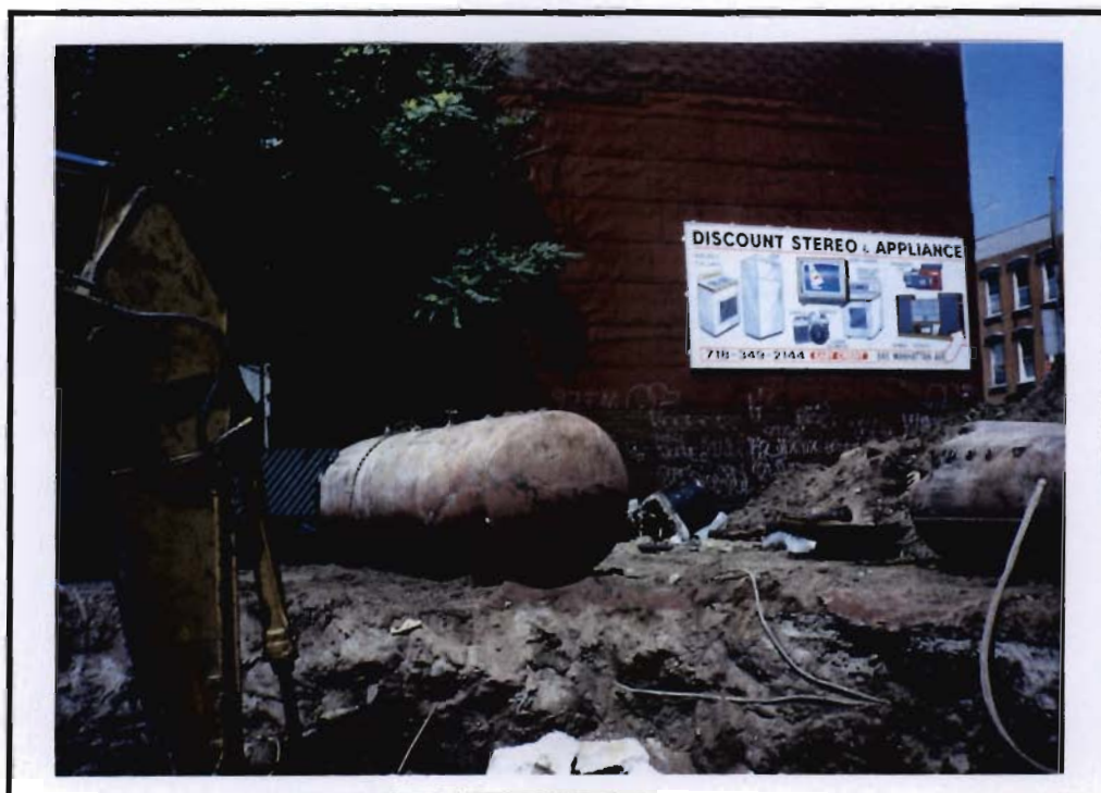
Two 4,000-gallon gasoline underground storage tanks
