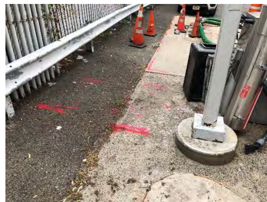
Photo of the vent pipes in pink
