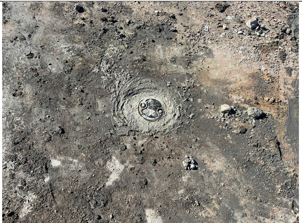
Photo 2 – Representative photo of a finished ground water monitoring well.
