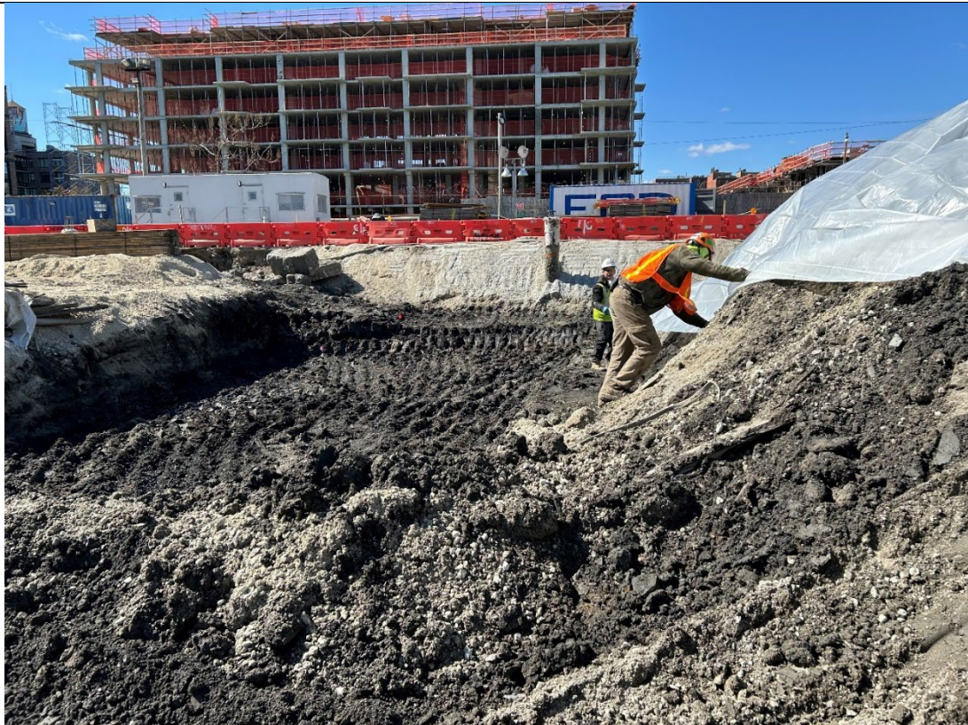
Photo 6 – Representative photo of excavation within grid F3 as well as poly sheeting placed over stockpile.
