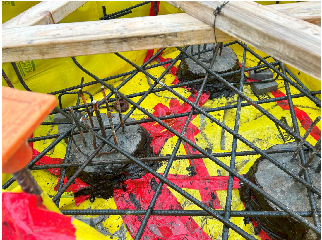
Photo 3 – Representative photo of Stego vapor barrier installation and footings. Note all overlaps were sealed with Stego Tape and all perforations sealed with Stego Mastic.
