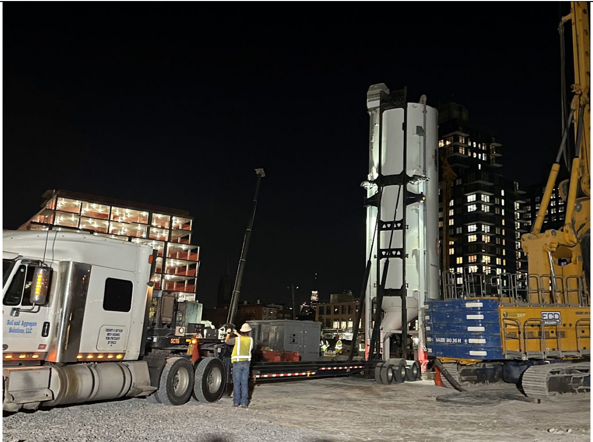
Photo 6 – Representative photo of Cascade mobbing ISS Pilot Test equipment during off-hours.
