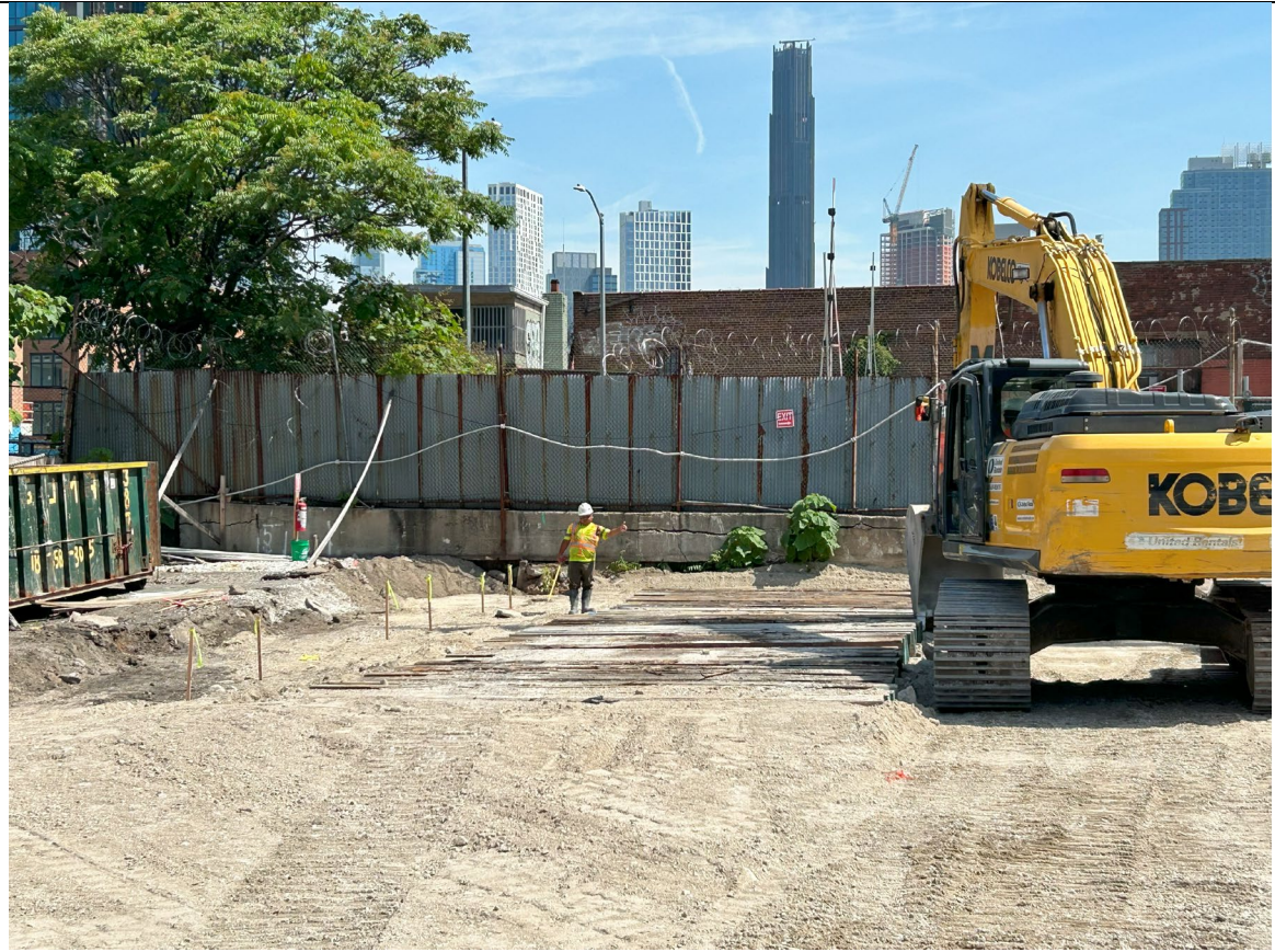
Photo 5 – Representative photo of ISS Pilot test area.
