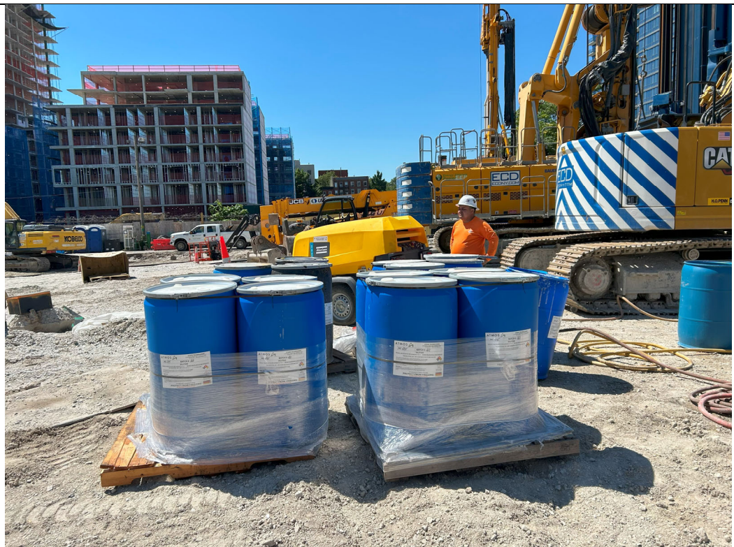
Photo 2 – Representative photo of ATMOS delivery.
