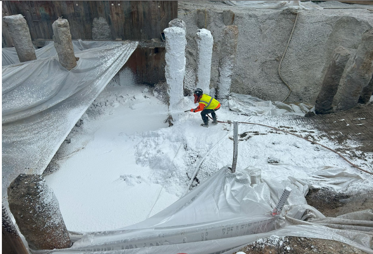
Photo 3 – Representative photo of preemptive spraying of ATMOS foam in Spill 2308807 area before excavation begins for offsite disposal.
