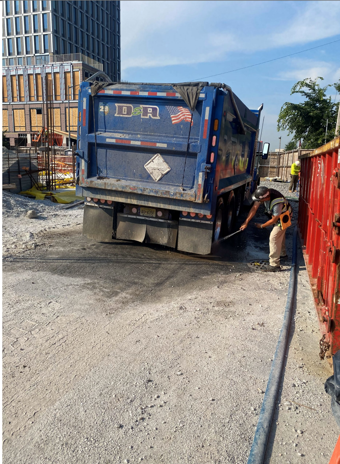
Photo 5 – Representative photo of truck sides tied down and tire washing prior to exiting the Site.
