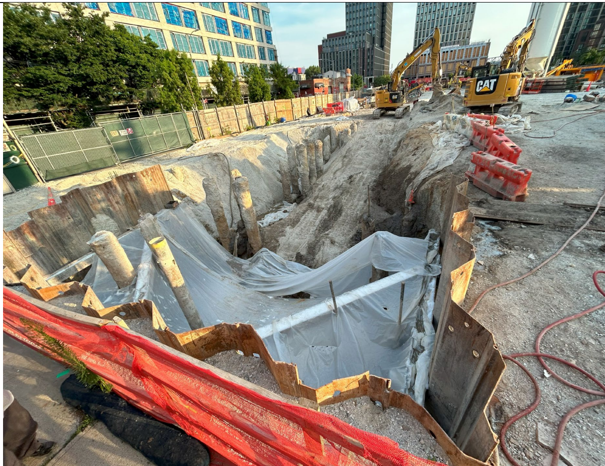
Photo 4 – Representative photo of Spill 2308807 excavated area sprayed with foam and covered with poly at the end of day.
