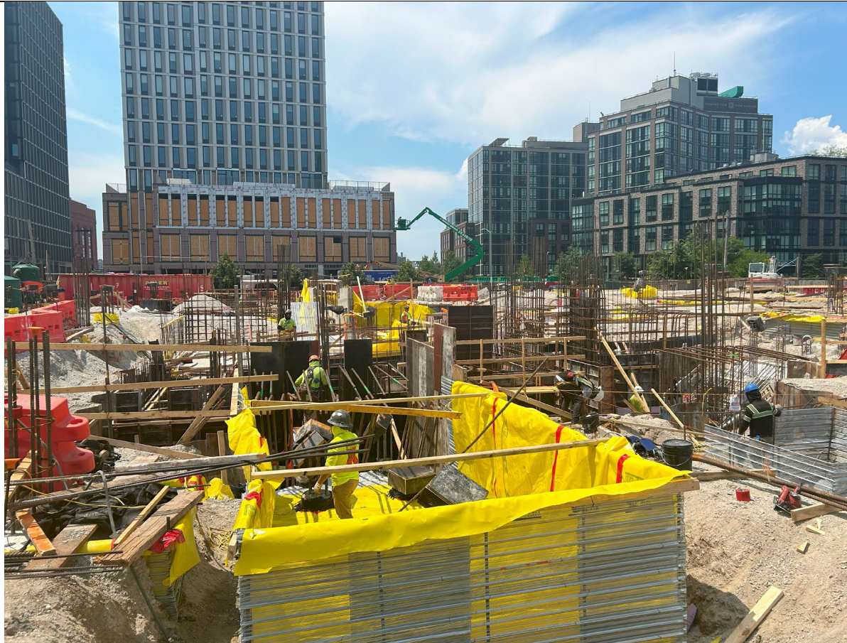
Photo 2 – Representative photo of vapor barrier and rebar installation in the south building.
