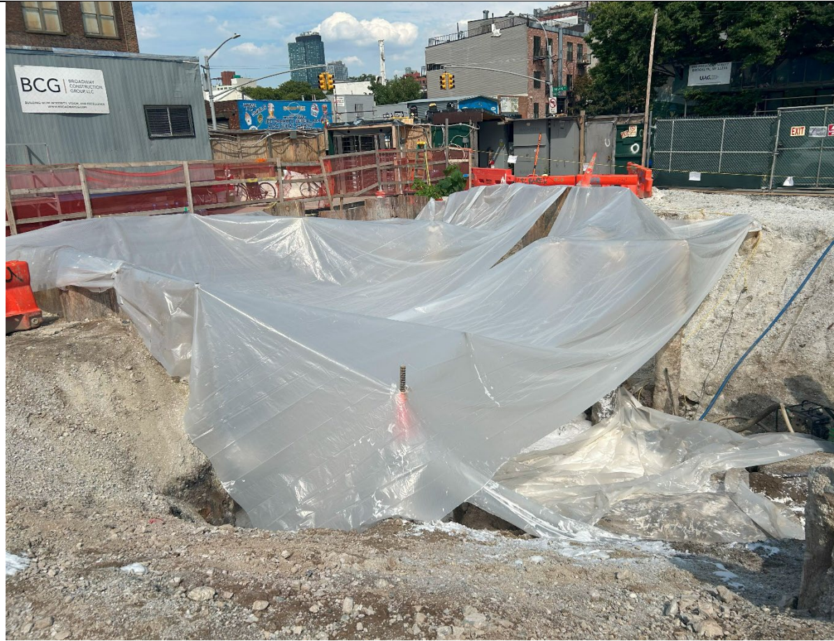
Photo 5 – Representative photo of spill 2308807 area covered with poly at the end of day.
