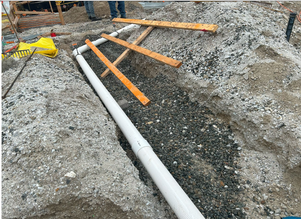
Photo 2 – Representative photo of SSDS installation in the south building.
