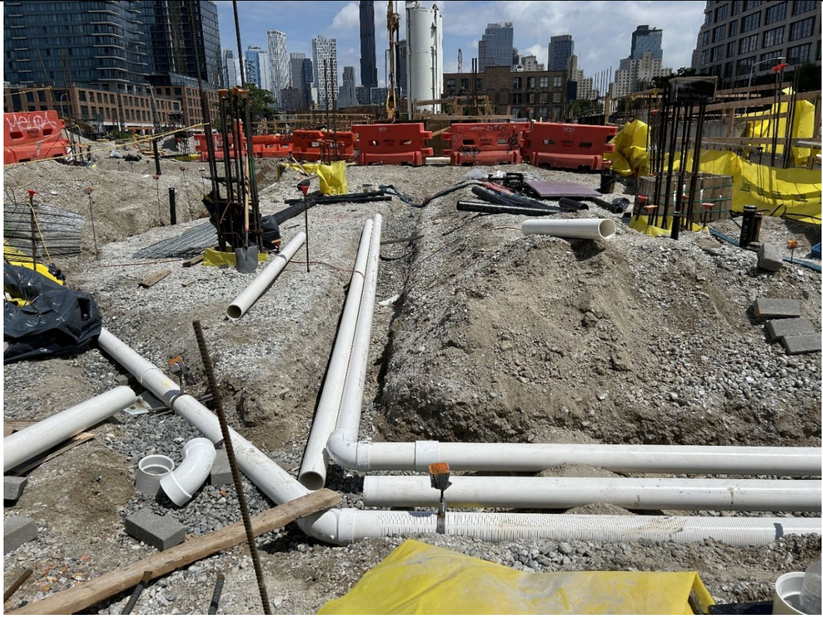
Photo 1 – Representative photo of SSDS piping installation.
