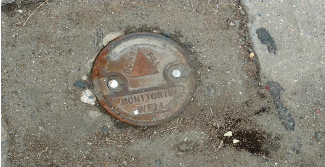
Photo 13: View of a groundwater monitoring well installed in the Flatlands Avenue sidewalk adjacent to the north of the subject property.
