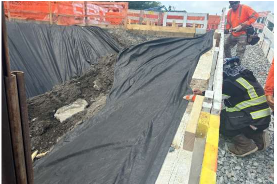
Photo 3 – United placing filter fabric above exposed soil in the southeastern portion of the Site, facing west.
