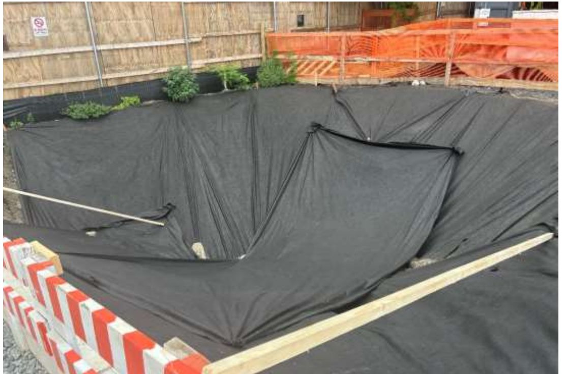
Photo 4 – Filter fabric placed above exposed soil in the southeastern portion of the Site, facing southeast.
