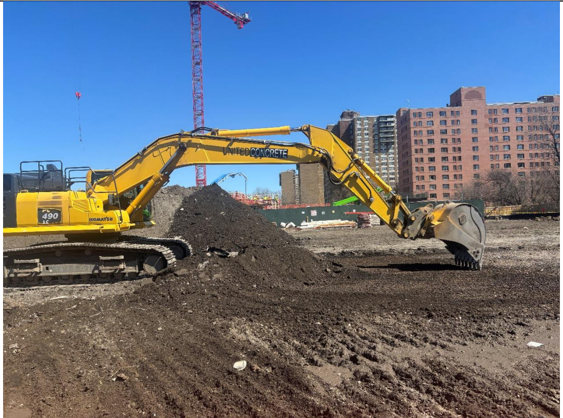
Photo 3 – United removing asphalt pavement in the eastern portion of the Site, facing east.
