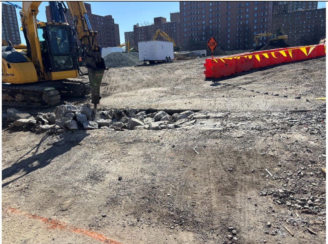
Photo 4 – United removing concrete above existing temporary electric lines in the northeastern portion of the Site, facing south.
